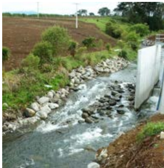
Incorporating a clear passage for fish when constructing the Kapuni water intake channel earned the South Taranaki District Council a TRC Environmental Award in 2014.
