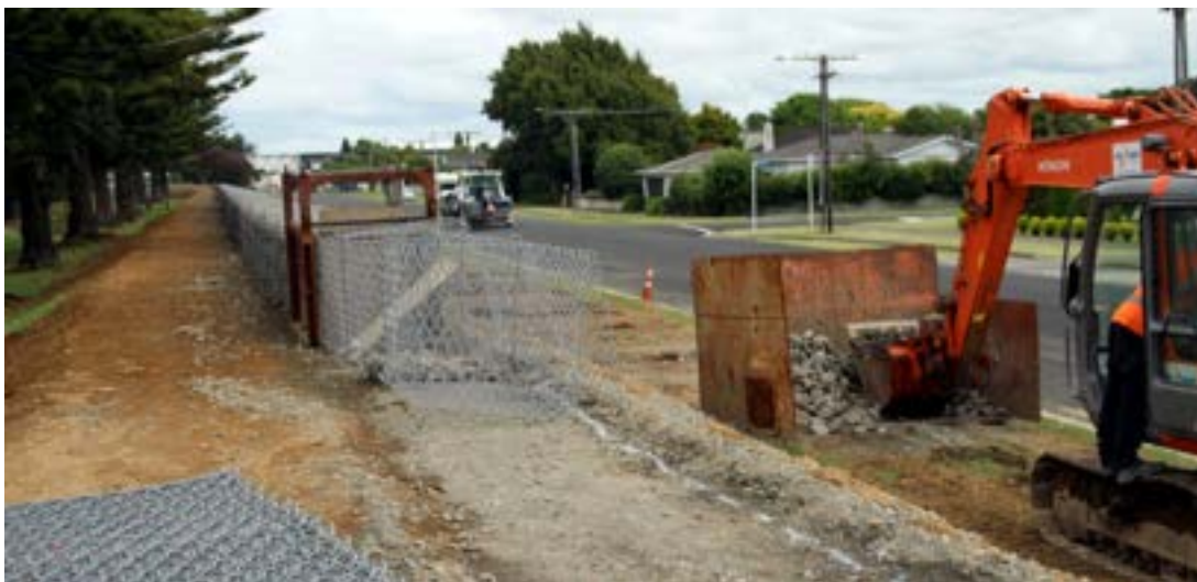
Flood protection work undertaken in Waitara includes the extension of flood banks.
