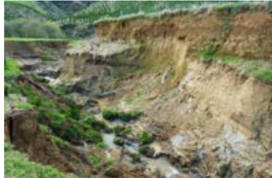
Heavy rain causes erosion and bank collapse in Mākāhu in the Stratford District.
