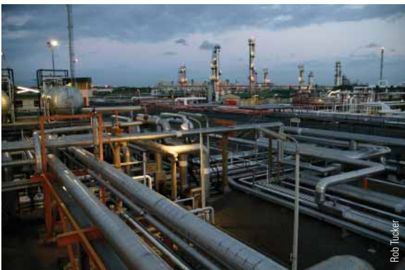
The Ōaonui Production Station processes gas from the Maui field.
