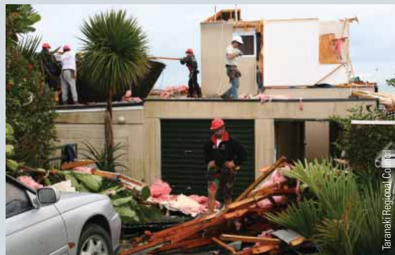
Clean-up operations after the 5 July tornado hit Ōākura.
