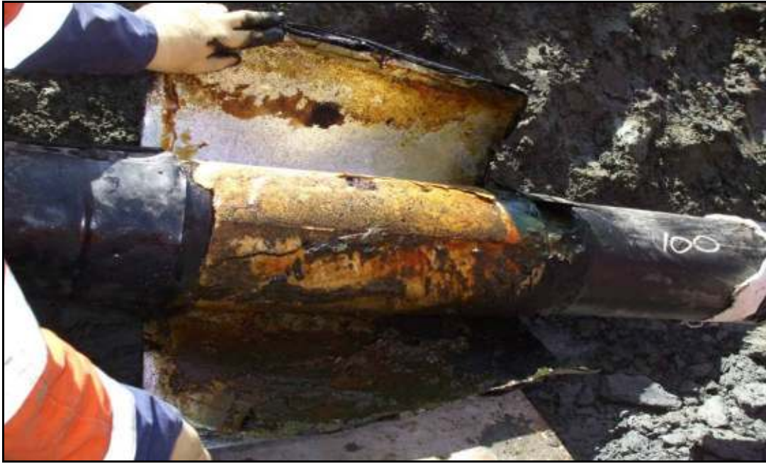
Photograph 10 – Exposed insulation section after wrap removal – 26 October 2010
