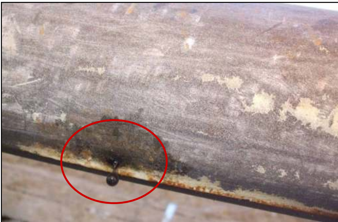
Photograph 14 - Location of the pipeline leak point - 8 November 2010
