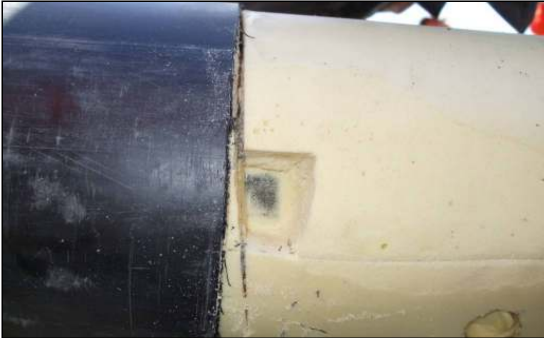
Photograph 9 – Exposed section of pipeline insulation – 22 October 2010
