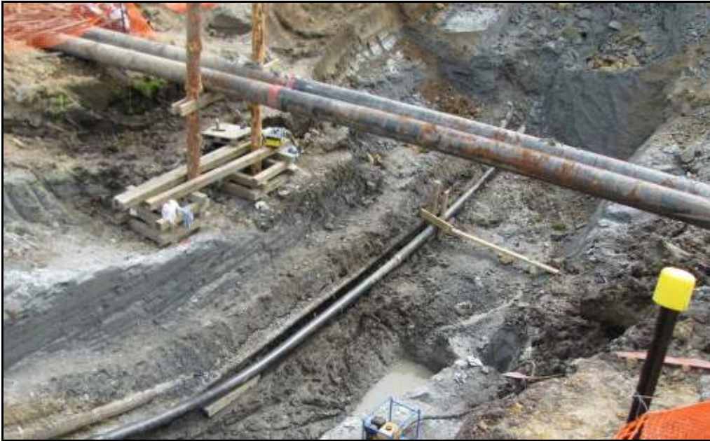
Photograph 13 – Tributary diversion above the oil pipe – 4 November 2010
