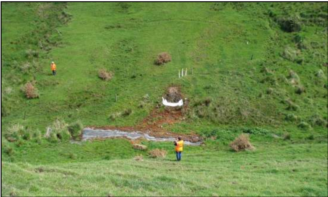
Photograph 2 – Inspecting the affected area - 8 October 2010. Pipeline leakage point upslope of white sheet
