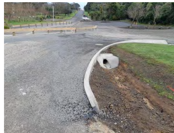
Shifting the entrance to the Hawera Cemetery due to existing intersection having a very poor sight visibility.
