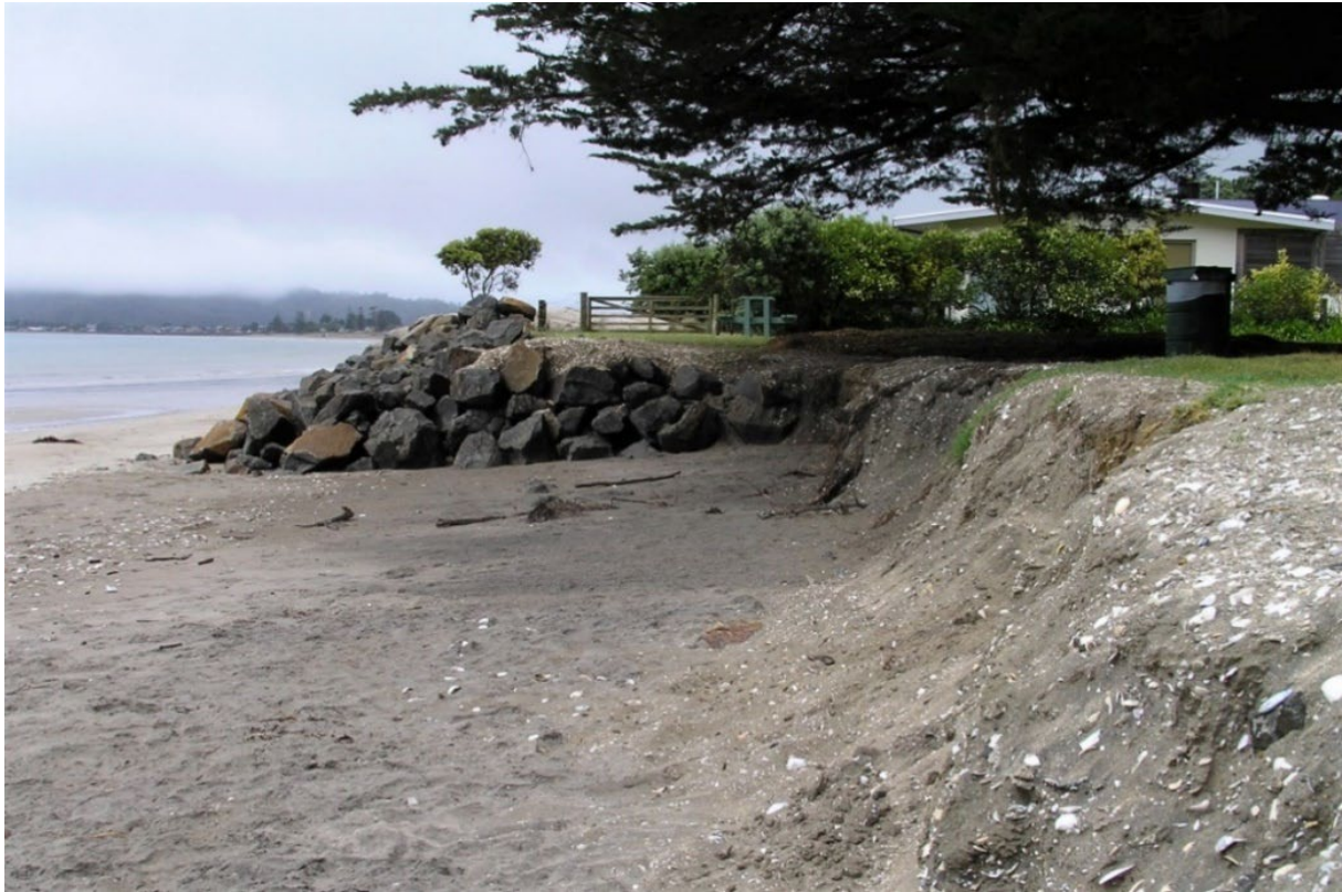
Figure 5-3: Erosion beside a sea wall in Whitianga. Credit: R. Bell, NIWA.
