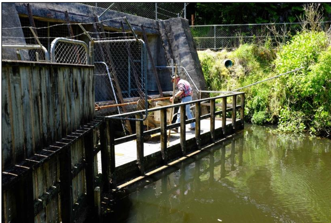
Figure 8. Mangorei HEPS intake to penstocks at Lake Mangamahoe.
