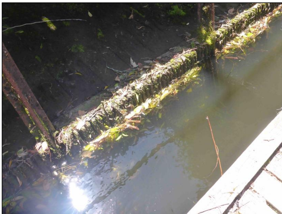
Figure 11. Mangorei HEPS intake trash screen on Lake Mangamahoe.
