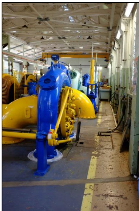
Figure 12. Mangorei HEPS Francis turbines.
