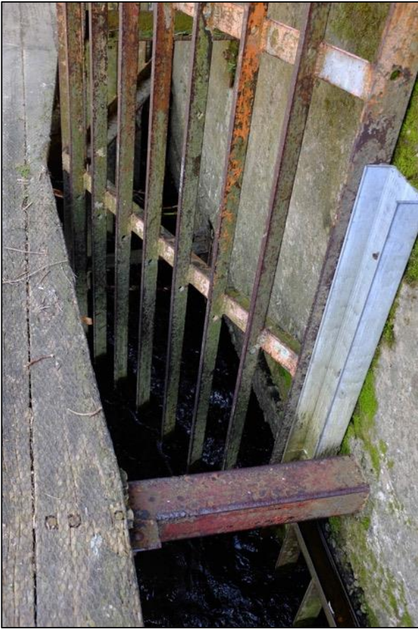
Figure 5. Mangorei HEPS Waiwhakaiho River intake gate trash rack.
