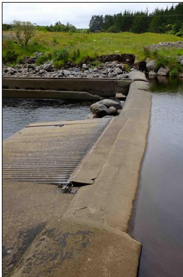
Figure 2. Mangorei HEPS low-head weir on the Waiwhakaiho River. Part of the fish pass can be seen in the background.
