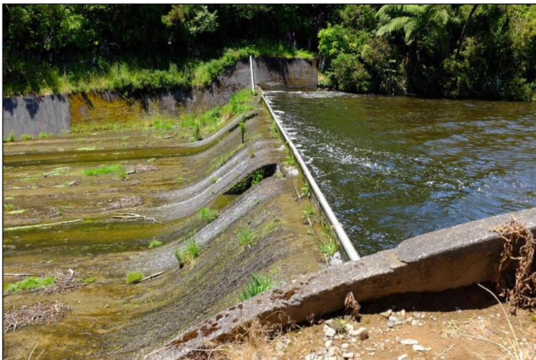
Figure 7. Standing on the Lake Mangamahoe earth dam looking towards the concrete spillway.
