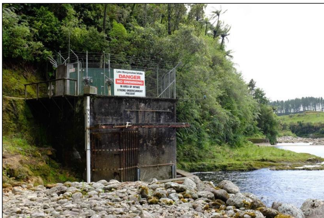
Figure 3. Mangorei HEPS intake structure on the Waiwhakaiho River.
