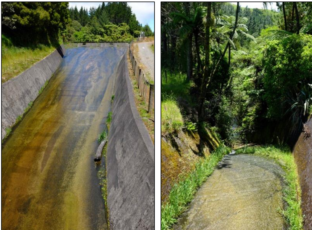
Figure 15. Lake Mangamahoe spillway looking up towards the lake (left) and down towards the Mangamahoe Stream (right).
