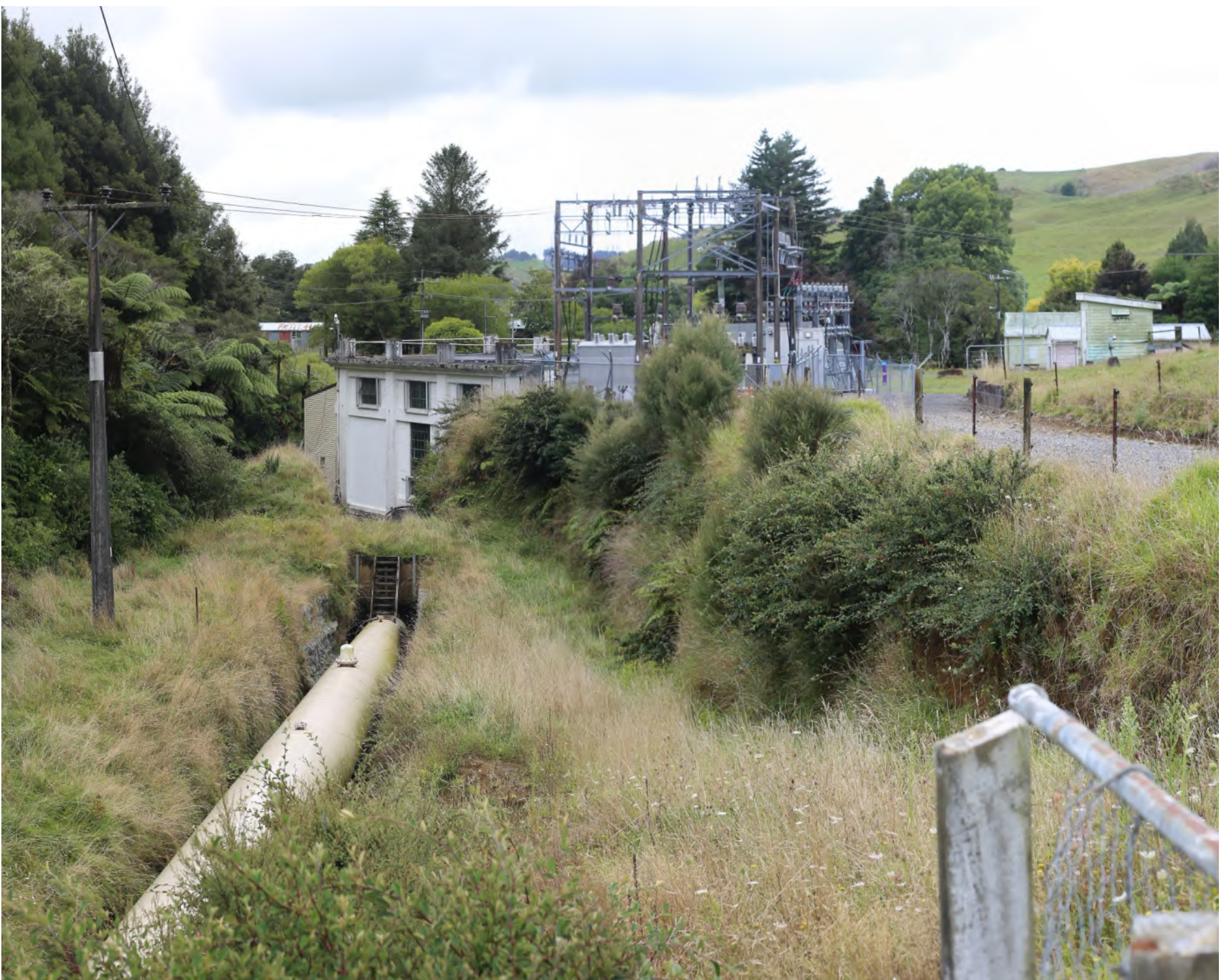
Penstock Above Power Station
