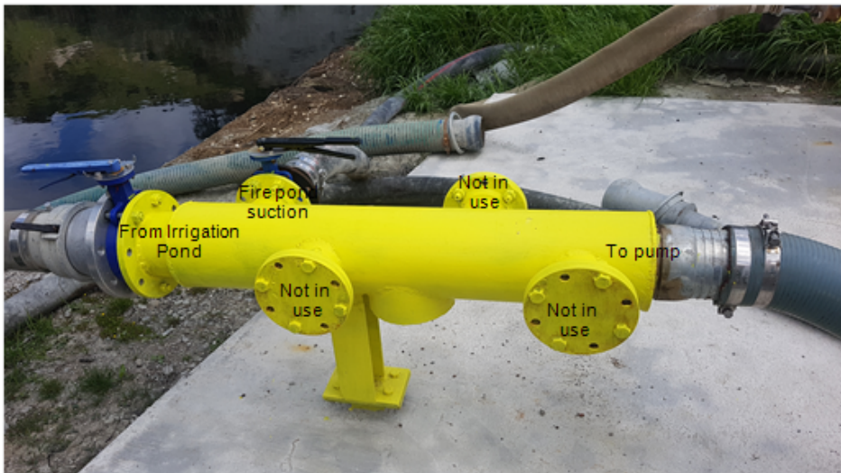
Pump Suction Manifold
