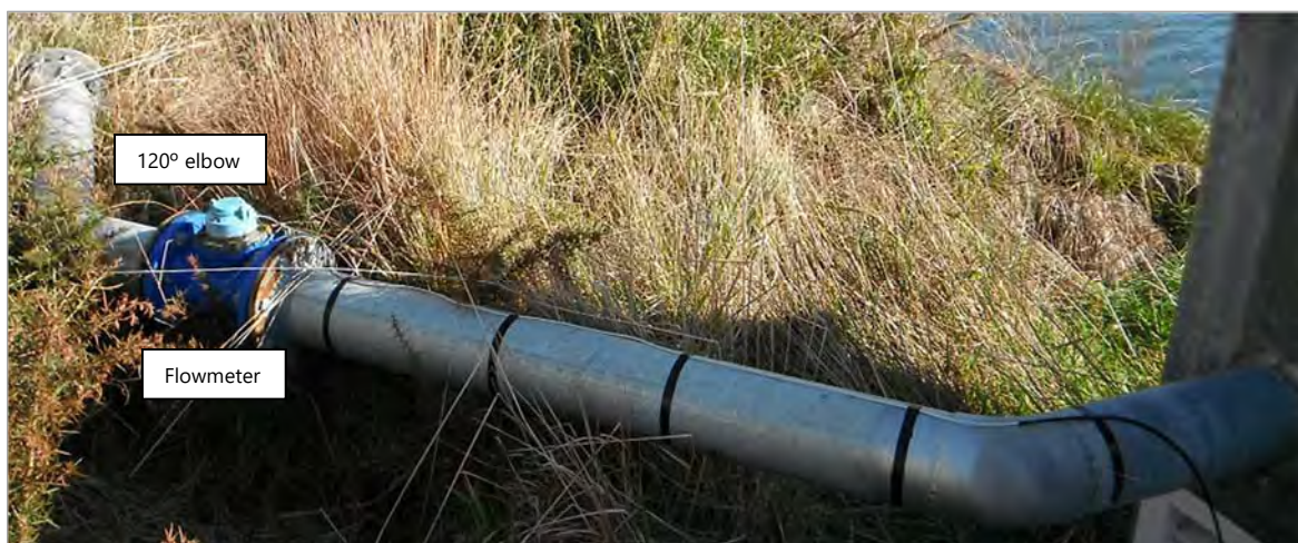
Photo 5 An example of a poor flowmeter installation
