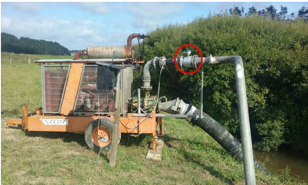
Photo 5 Poor installation of a flowmeter
