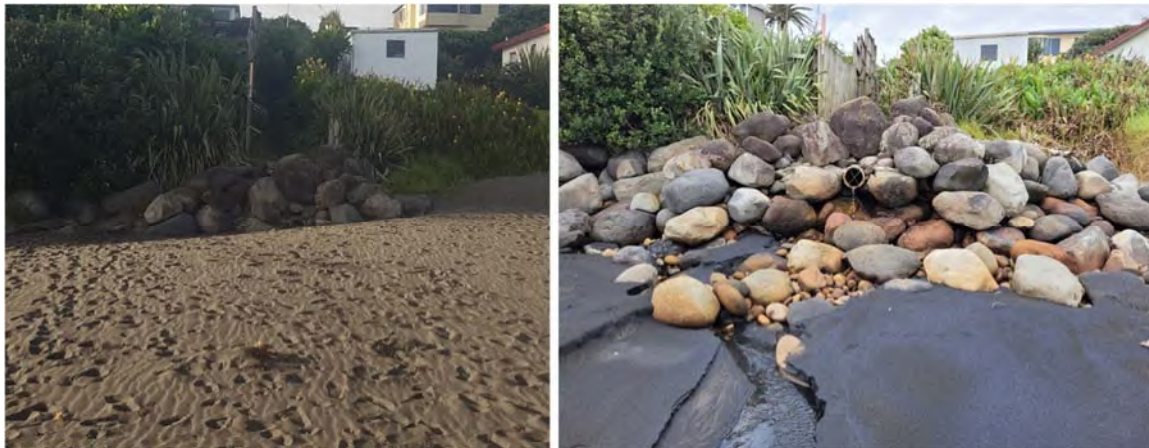
Photo 1 Beach level significantly higher in April 2020 (left), compared to June 2022 (right) at the Messenger Terrace stormwater outfall
