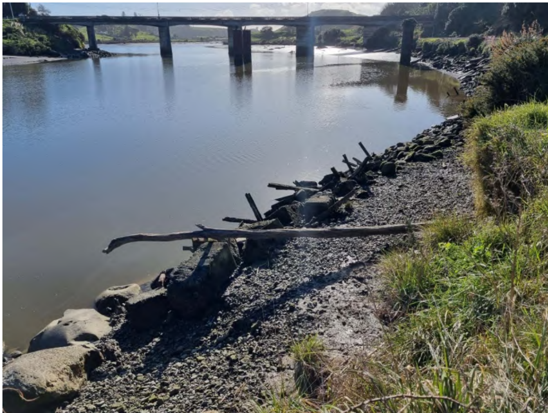
Photo 22 Posts protruding from rip-rap upstream of wharf (13 June 2023)
