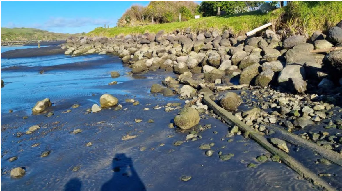
Photo 19 Rock wall downstream of boat ramp showing displaced rocks (13 June 2023)
