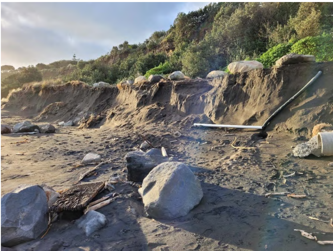
Photo 9 Increased erosion adjacent to Middleton Bay seawall showing hazardous boulders on the scarp (29 June 2021)
