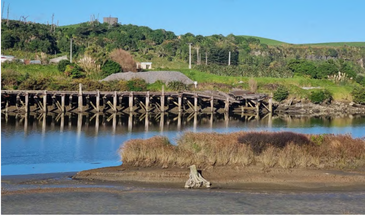
Photo 23 Collapsing section of Pātea wharf (13 June 2023)
