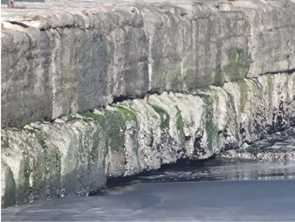
Photo 17 Northern mole showing scouring underneath (13 June 2023)
