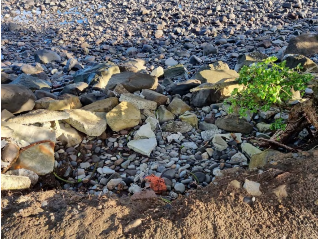
Photo 8 Unsuitable fill materials below picnic table and pine trees (13 June 2023)
