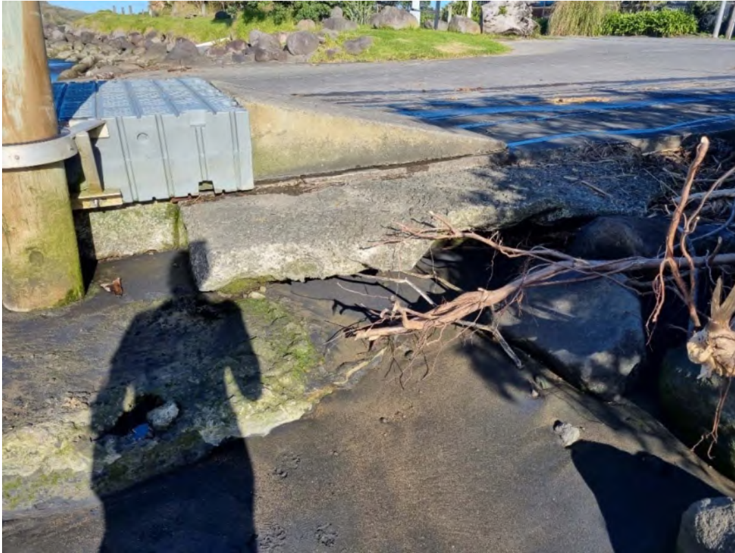
Photo 18 Pātea jetty showing scouring underneath (13 June 2023)
