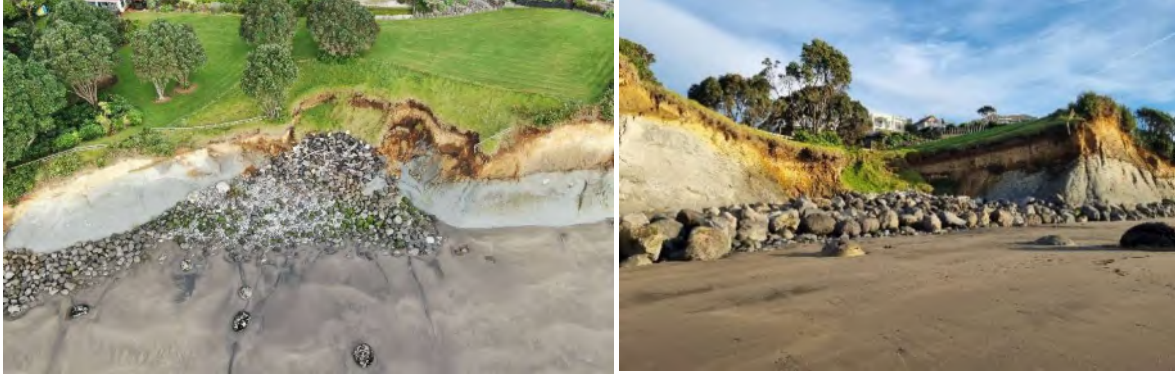
Photo 8 Onaero Beach rock rip rap incision repairs, June 2021 (left) and June 2024 (right)
