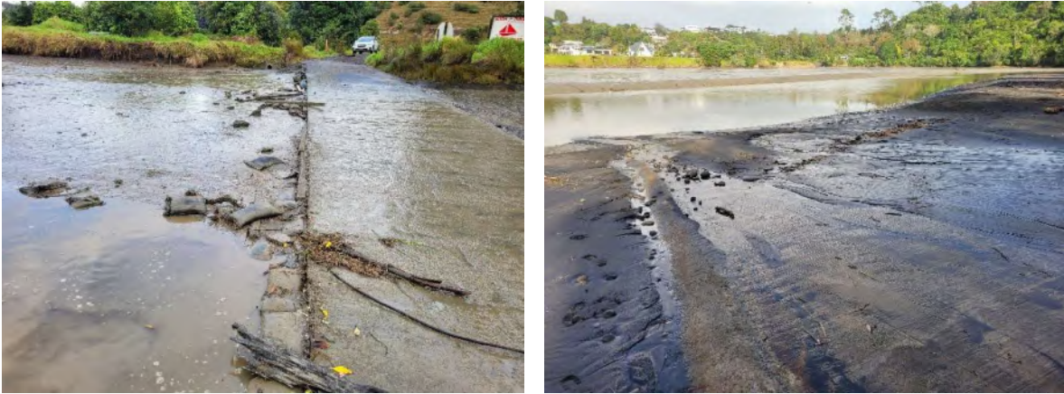
Photo 2 Displaced sandbags at the Tongaporutu boat ramp (left), and sand deposition on the Urenui boat ramp (right), 8 June 2024
