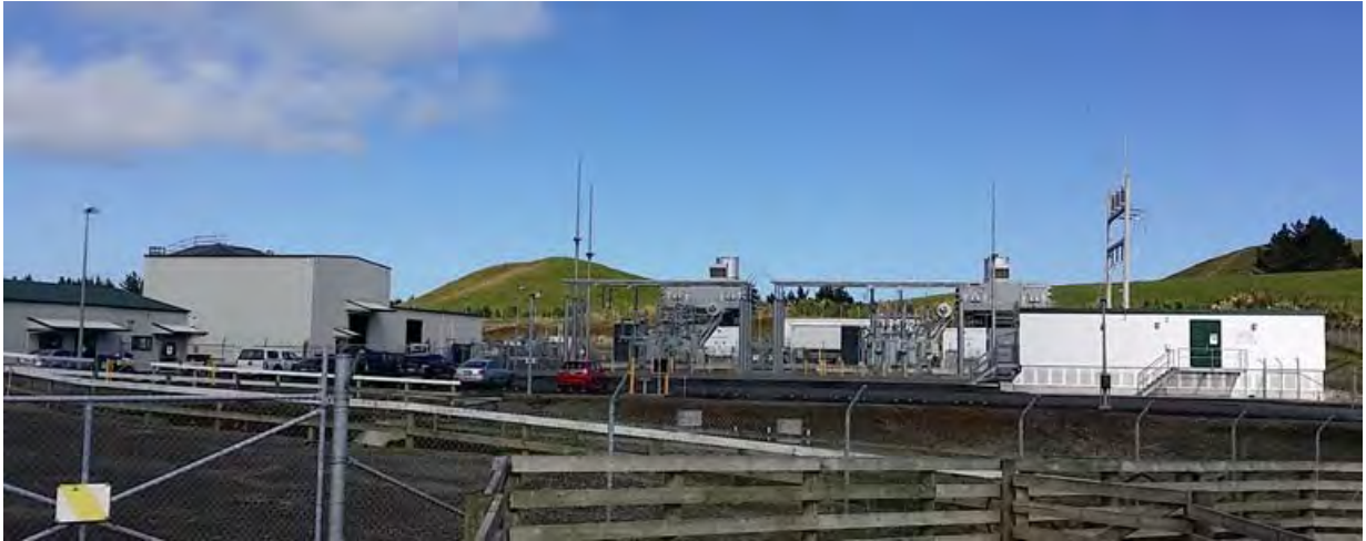
Photo 1 Nova McKee Power Plant
