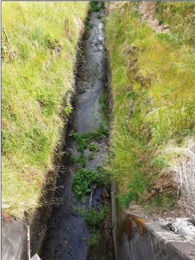
Photo 2 Old sluice gate leak (top) and race (bottom). Photos in 2019-2020 compliance period
