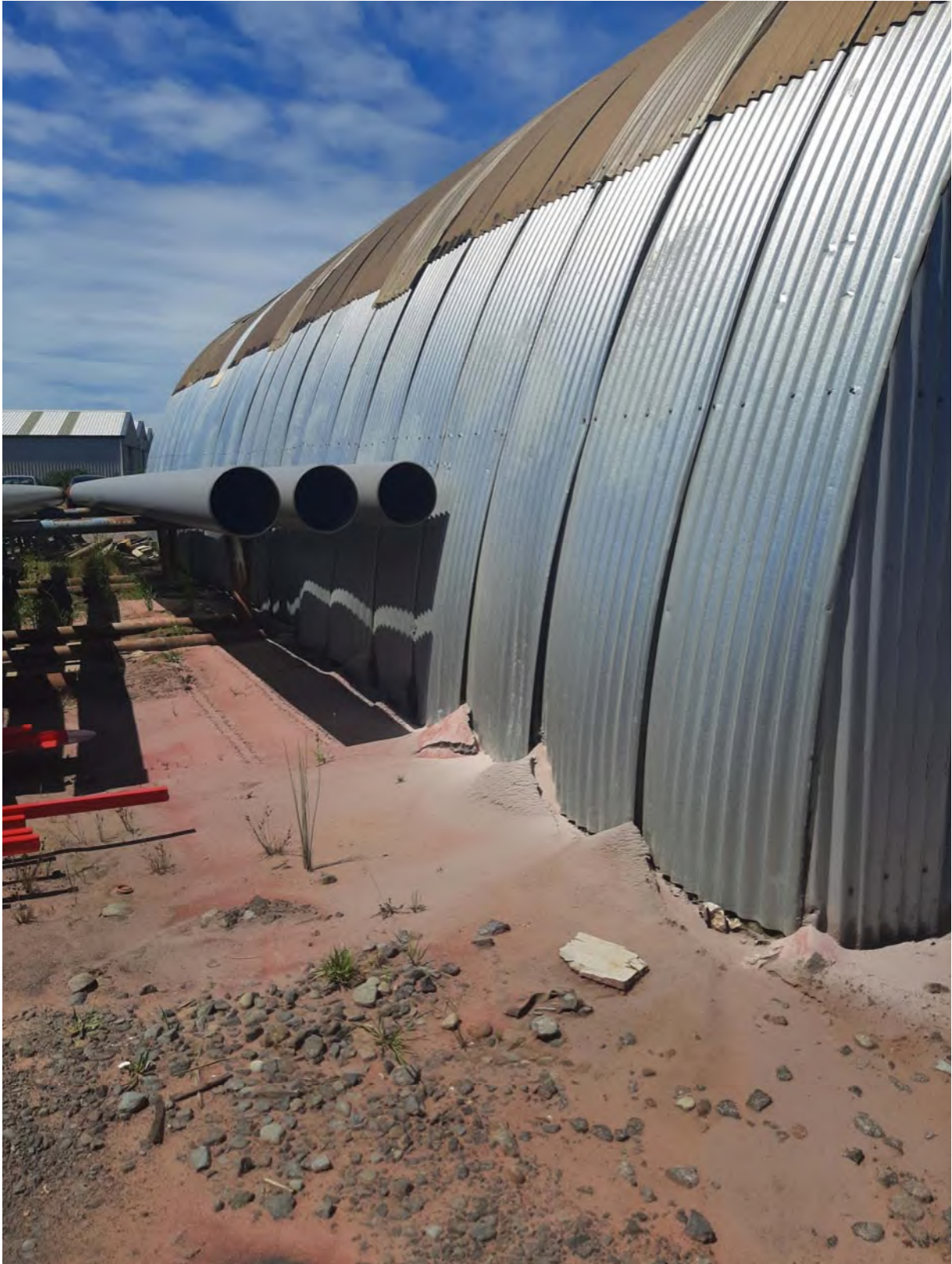
Photo 3 Material escaping from blasting shed, 9 February 2022
