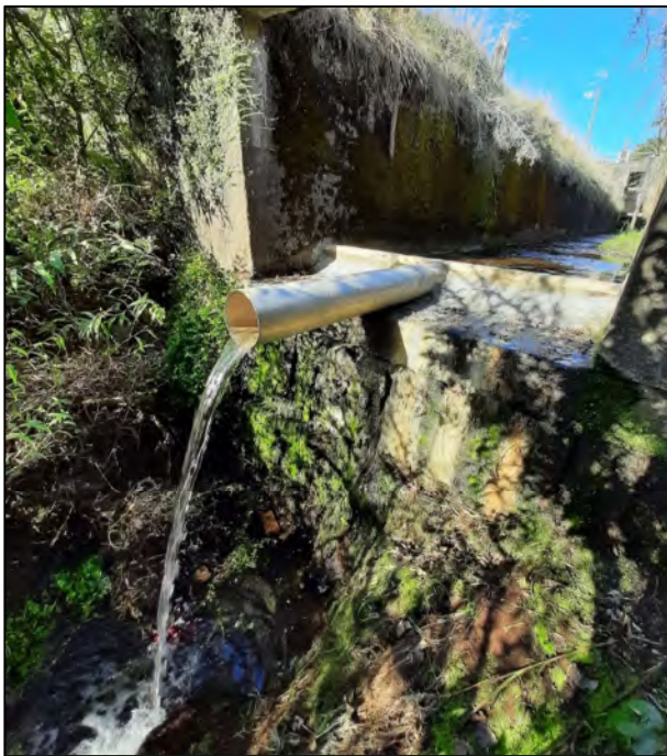
Photo 3 Installed perched pipe at outlet of sluice channel aimed at removing attractant flow for climbing fish (April 2022)
