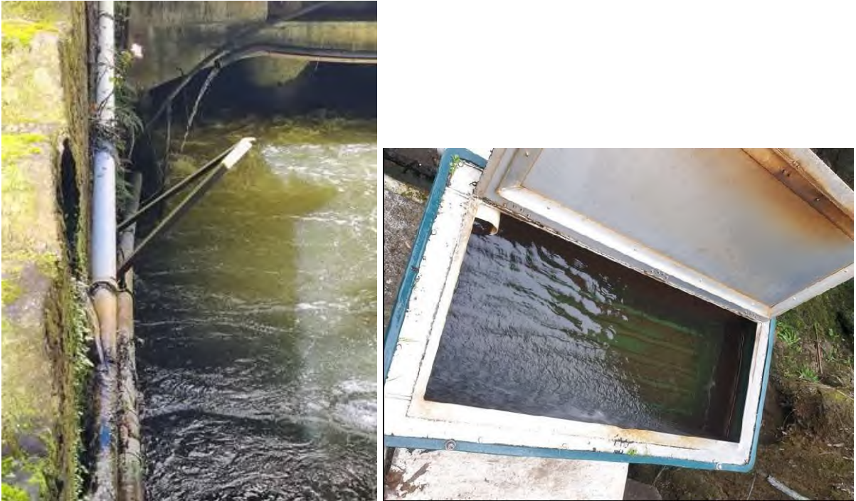
Photo 5 Attractant flow and piping to the elver trap (left (2023)). Elver trap at the station (right (2019))
