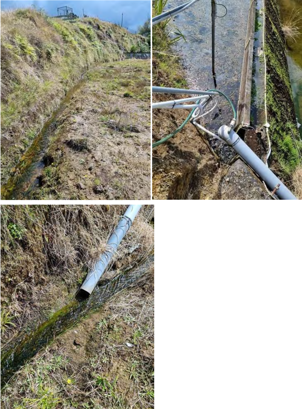
Photo 4 Fish pass at spillway (top right). Fish pass inlet (top left). Fish pass approach through spillway (bottom left (2023/24))
