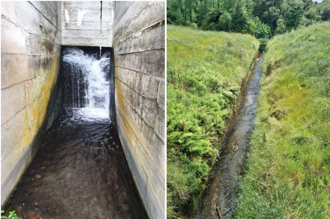
Photo 2 Old sluice gate leak (left (2019-2020)) and race (right (2022/23))
