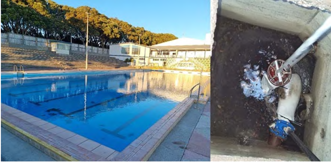
Photo 2 Todd Energy Aquatic Centre outdoor pool and muslin cloths in place over outlet pipes (8 May 2024)
