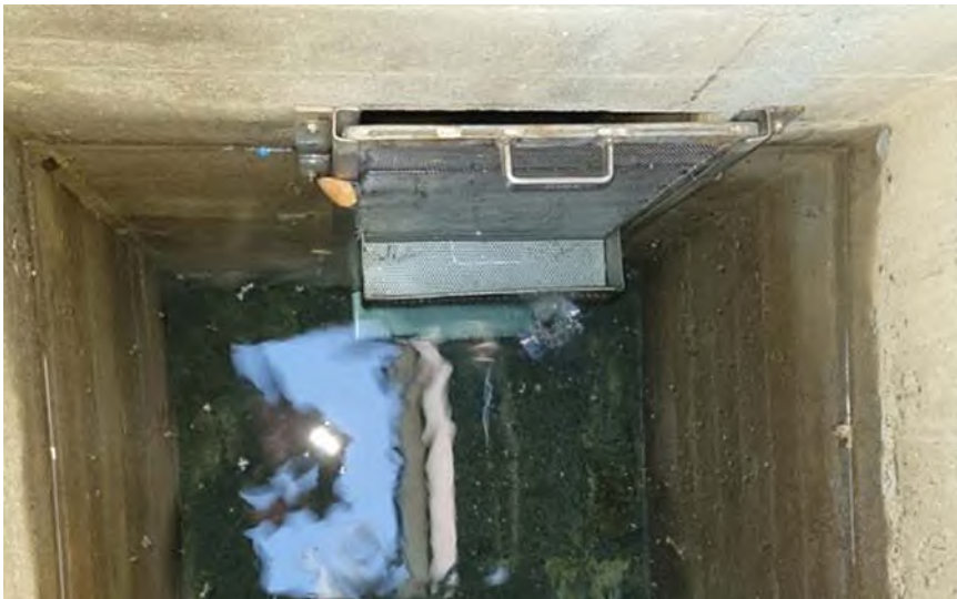
Photo 3 Additional debris screens in place in backwash holding tank at eastern end of the outdoor pool (8 May 2024)
