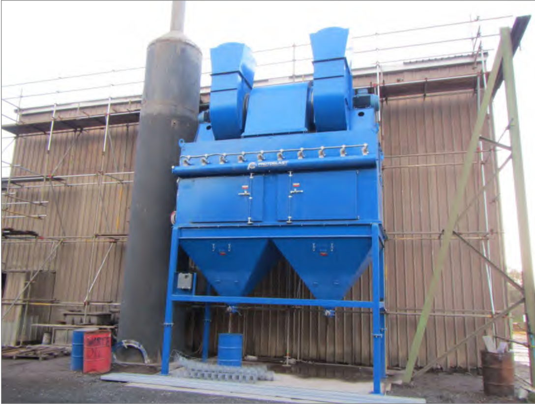
Photo 2 Blastquip fabric filter air treatment system at Dialog Fitzroy
