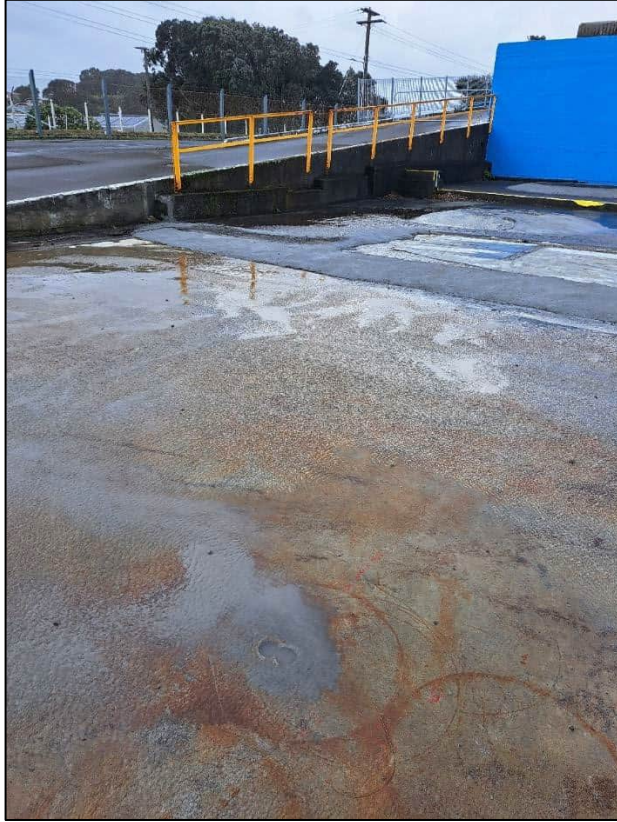
Photograph 5: Former storage of round drums on the concrete adjacent to Building 03.
