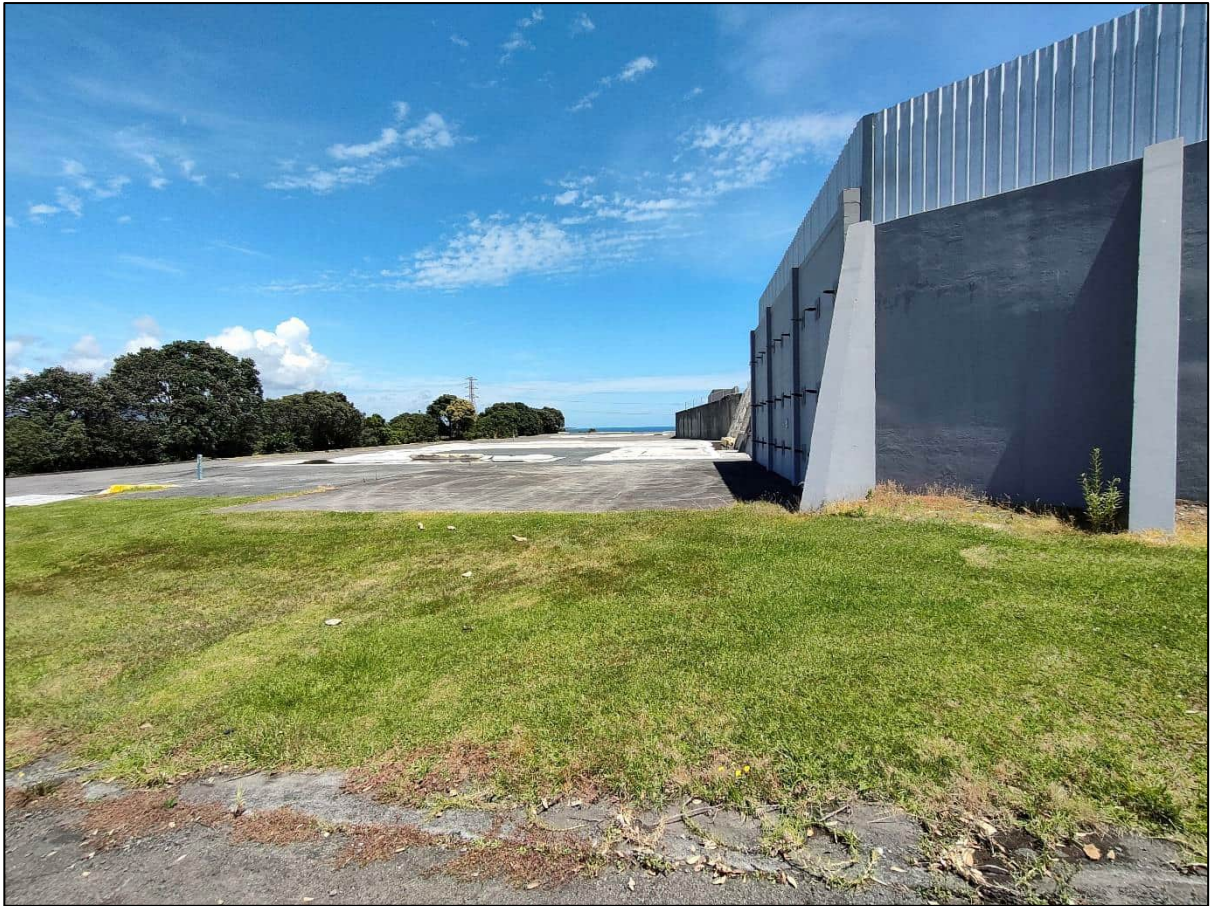
Photograph 7: View looking west showing the former footprint of Building 13, the retaining wall to the top yard behind Building 3.
