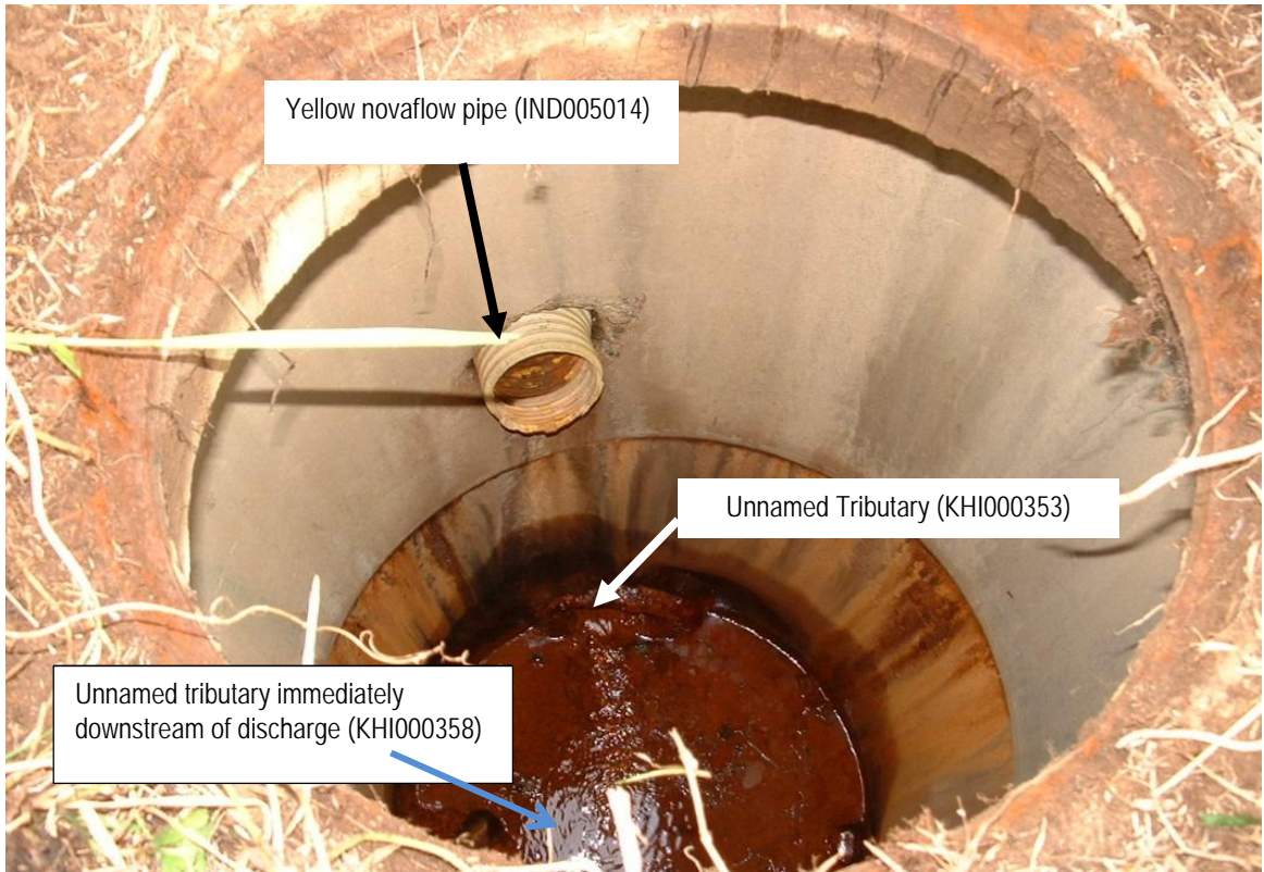
Photo 1 The view down manhole 1 including outlet of the unnamed tributary, the yellow novaflow pipe from the Taranaki Galvanizers site (IND005014) and the tributary immediately downstream of the discharge (KHI000358)
