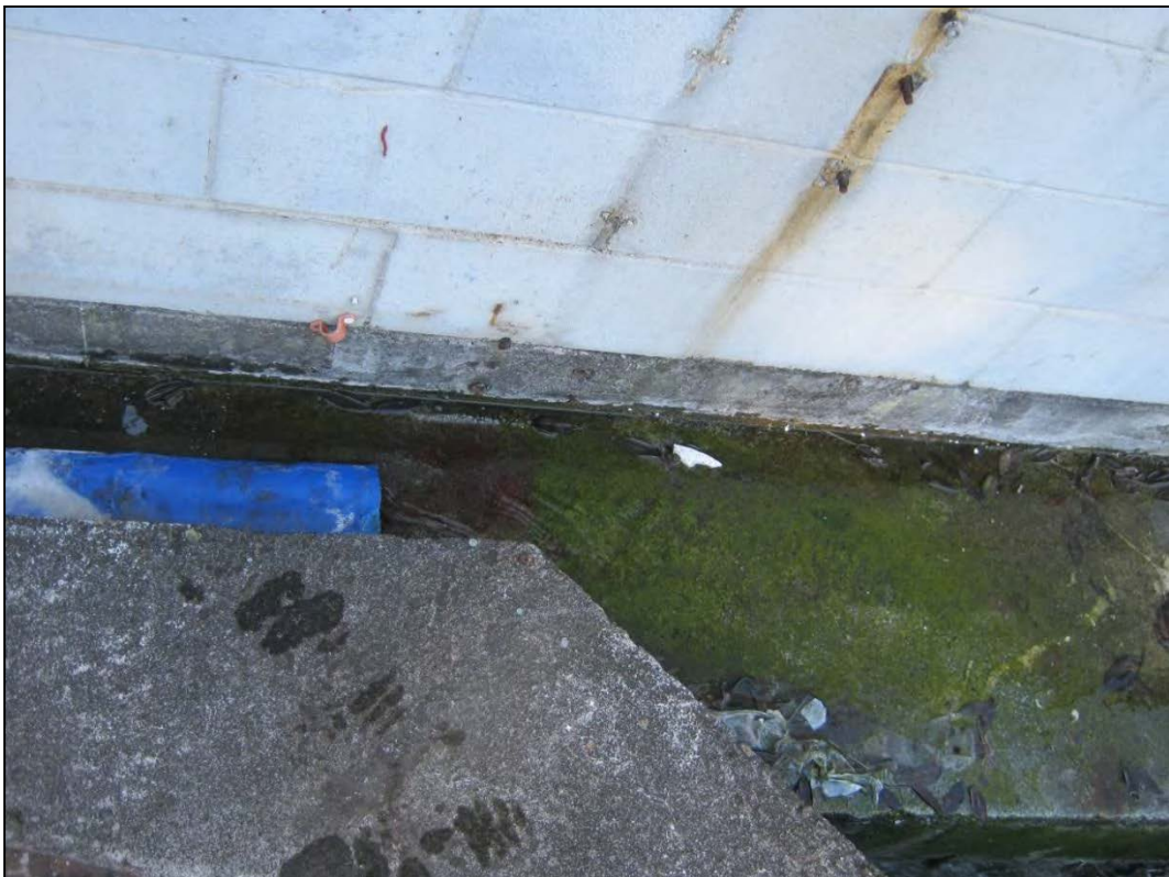
Photo 2 Oil cooling water sampling point
