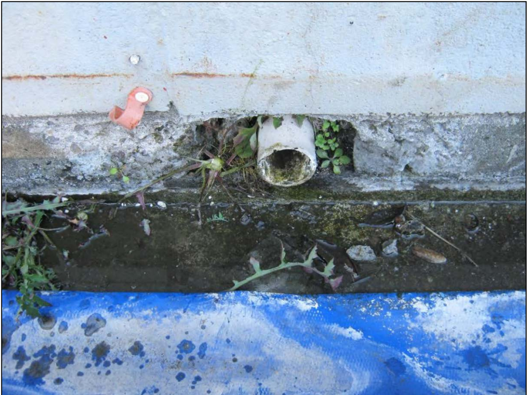
Photo 3 Cooling water from evaporative condenser sampling point
