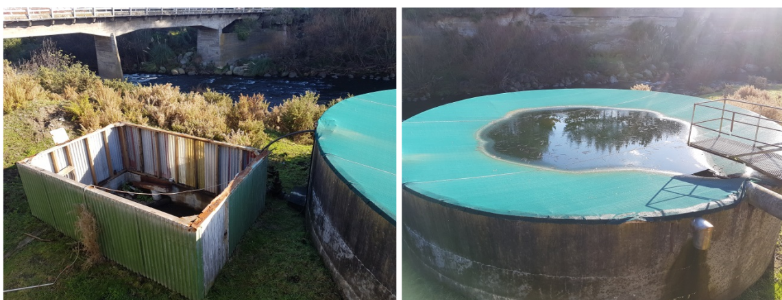
Photo 2 Left: Pump shed roof removed to access faulty pump. Right: Holding tank at capacity. 20 June 2016
