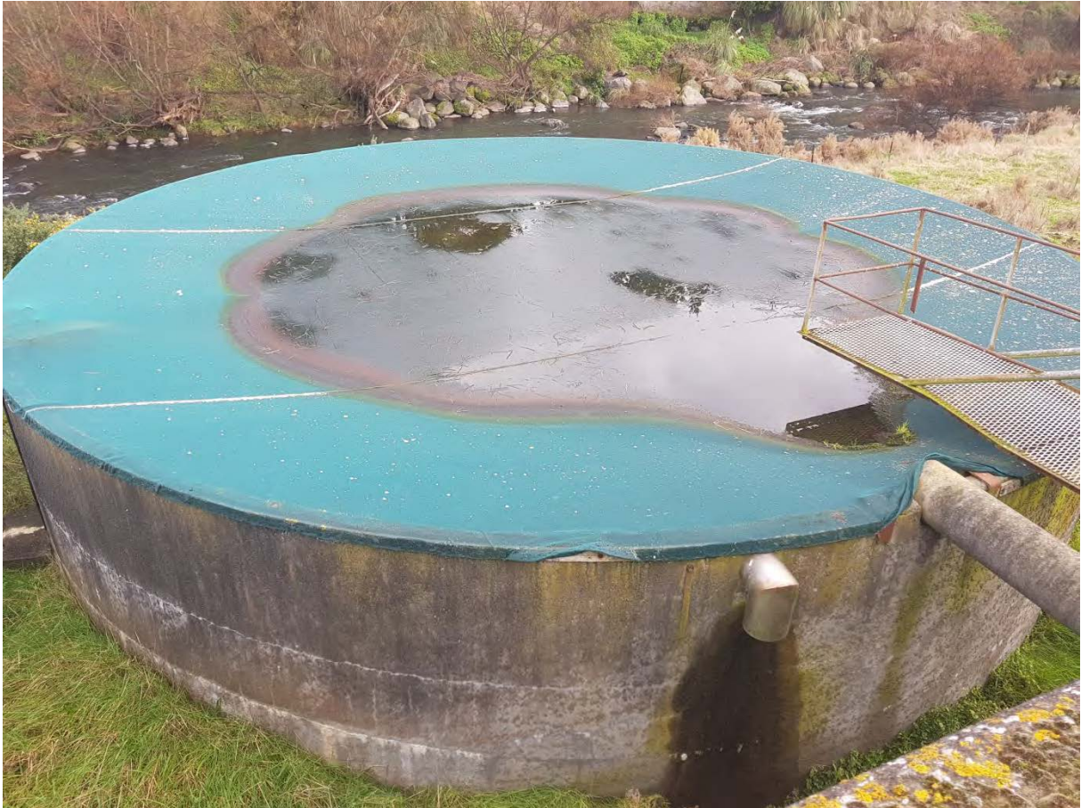
Photo 2 Water visible at the discharge pipe from previous overflow events (16 June 2017)
