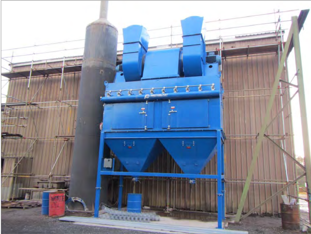
Photo 2 Blastquip fabric filter air treatment system at Fitzroy Engineering
