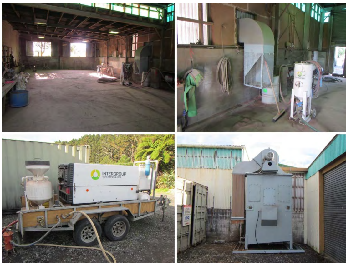
Photo 3 Site photos from Intergroup Ltd showing the blasting shed and key process equipment
