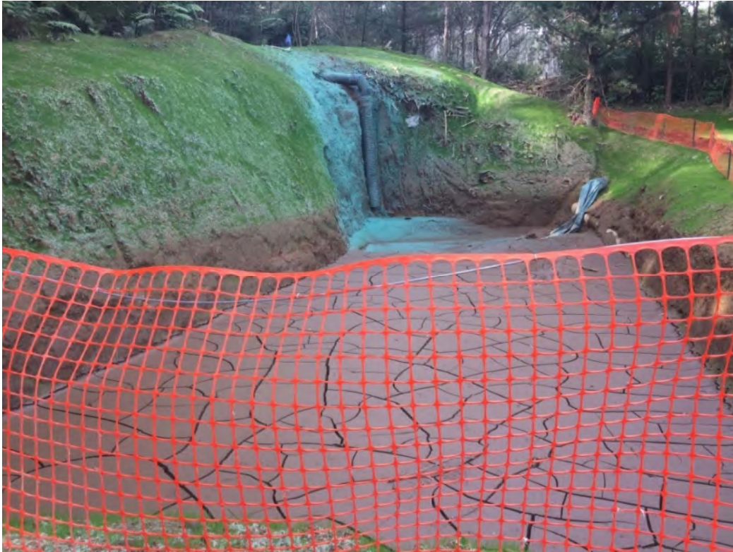
Photo 4 Pretreatment pond for large silt pond, May 2021
