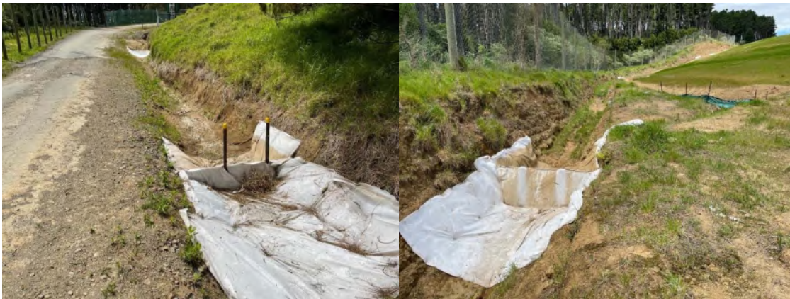
Photo 13 Examples of the type of weirs installed in the stormwater drains to retain sediment.
