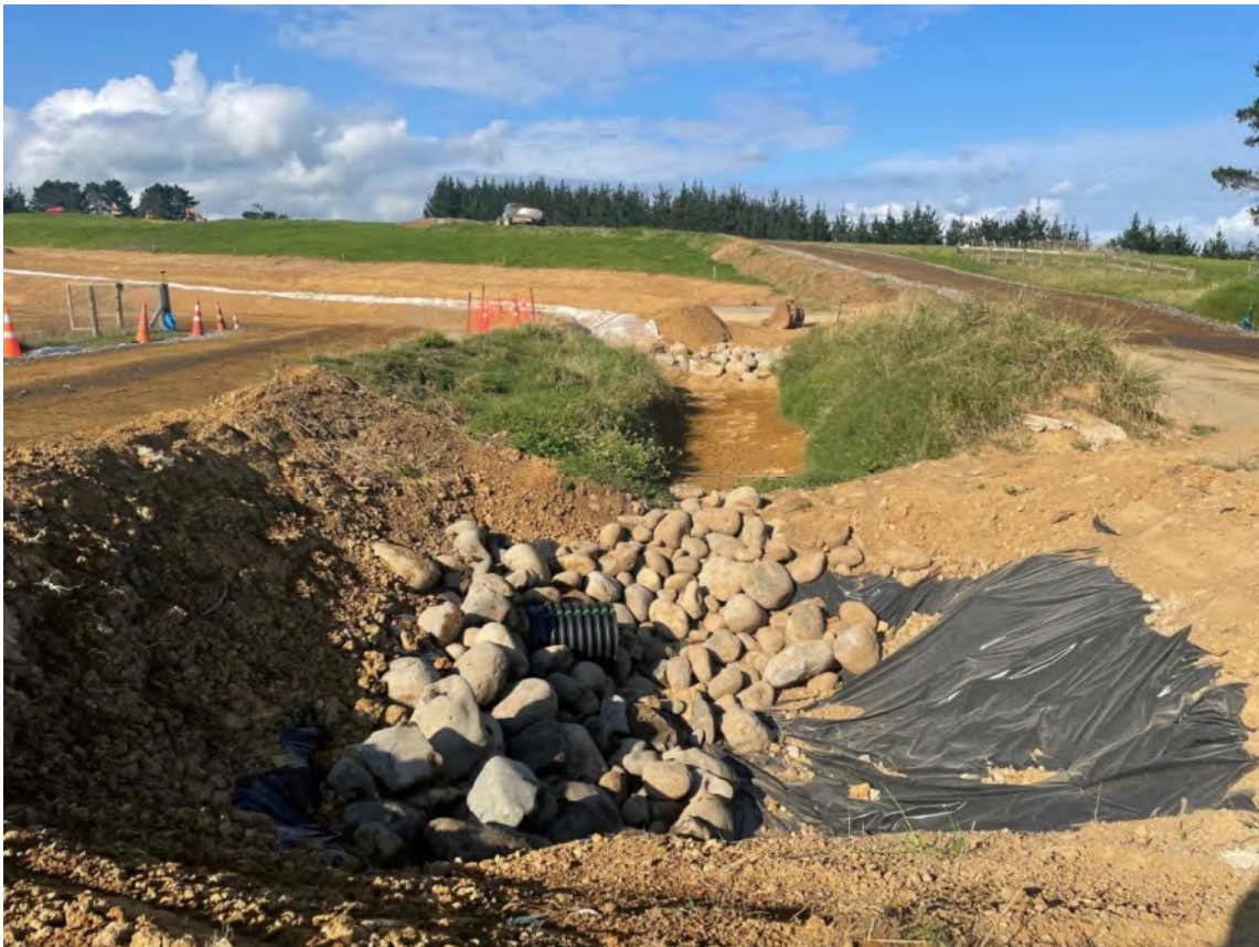
Photo 3 Amended drainage and access to enable capping works for Stage 2 remediation, March 2022
