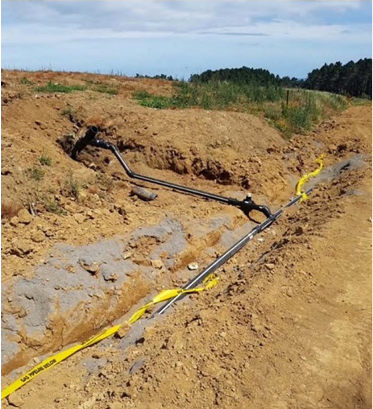
Photo 7 Leachate pipes feeding into the gas collection system
