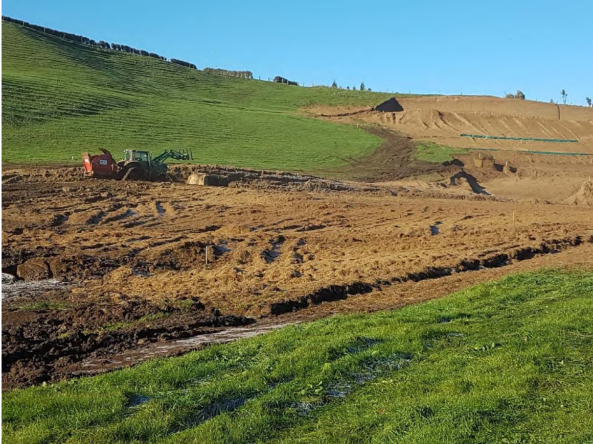
Photo 4 Central Landfill, 3 July 2018 – northern side of southern gully
