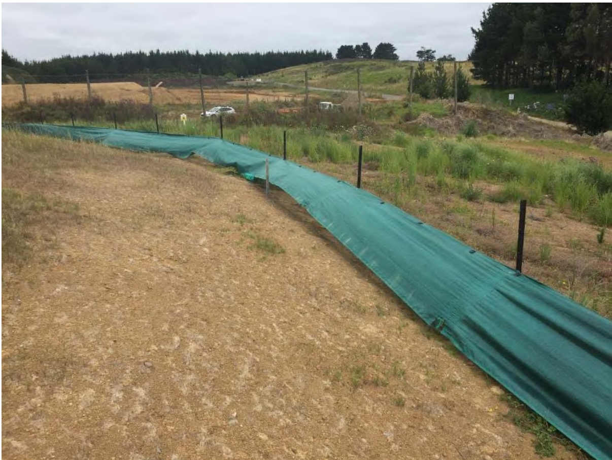
Photo 9 Example of incorrectly installed silt fence 27 January 2021
