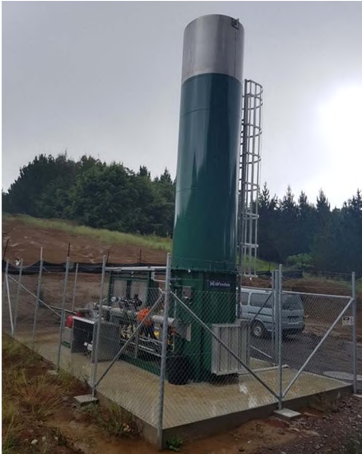
Photo 6 The fully enclosed flare
