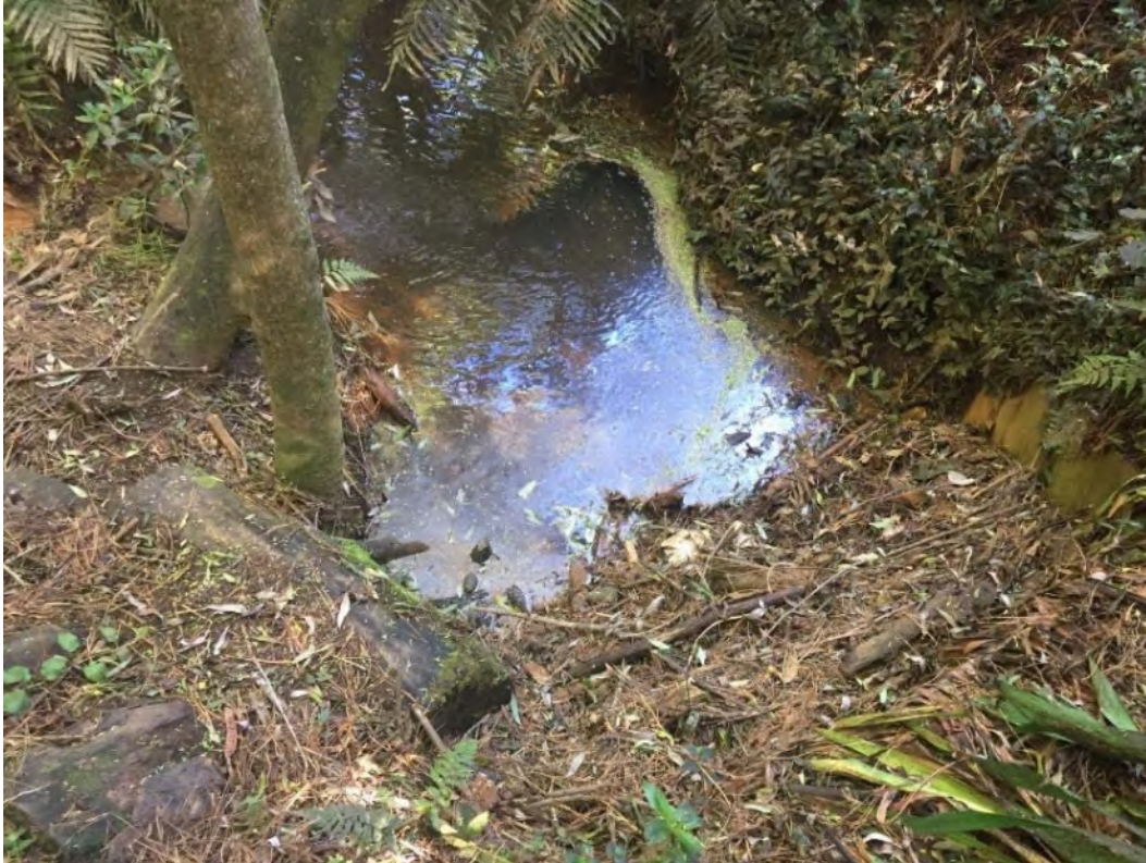
Photo 13 Accumulation of debris at the SPCA driveway culvert inlet, April 2021
