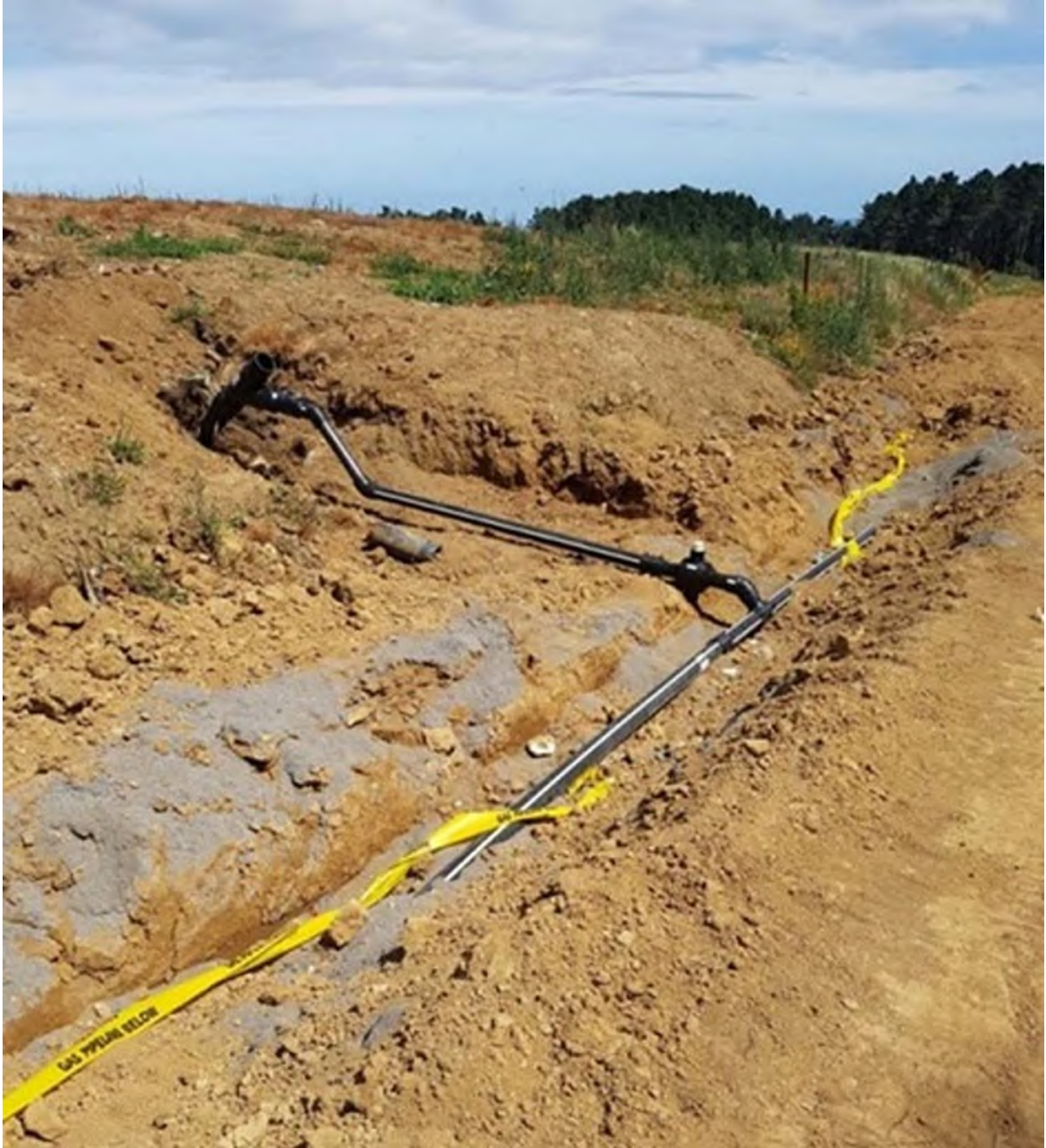
Photo 5 Leachate pipes feeding into the gas collection system
