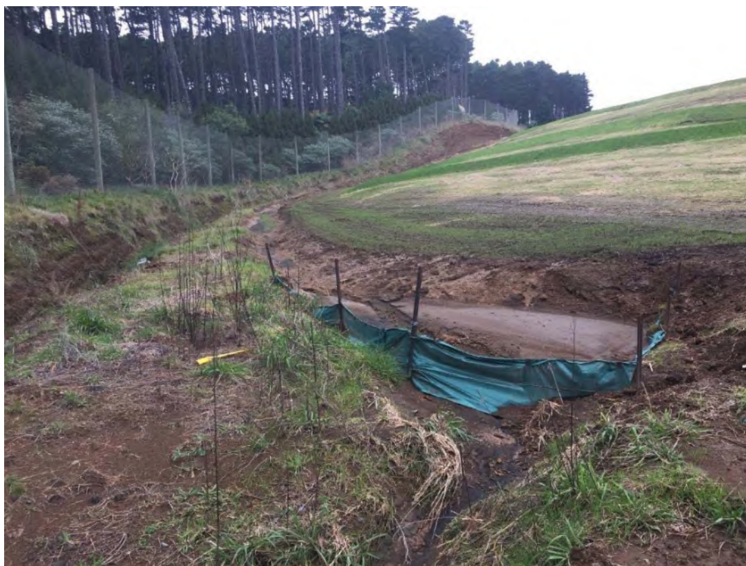
Photo 17 Silt fence requiring maintenance, June 2021
