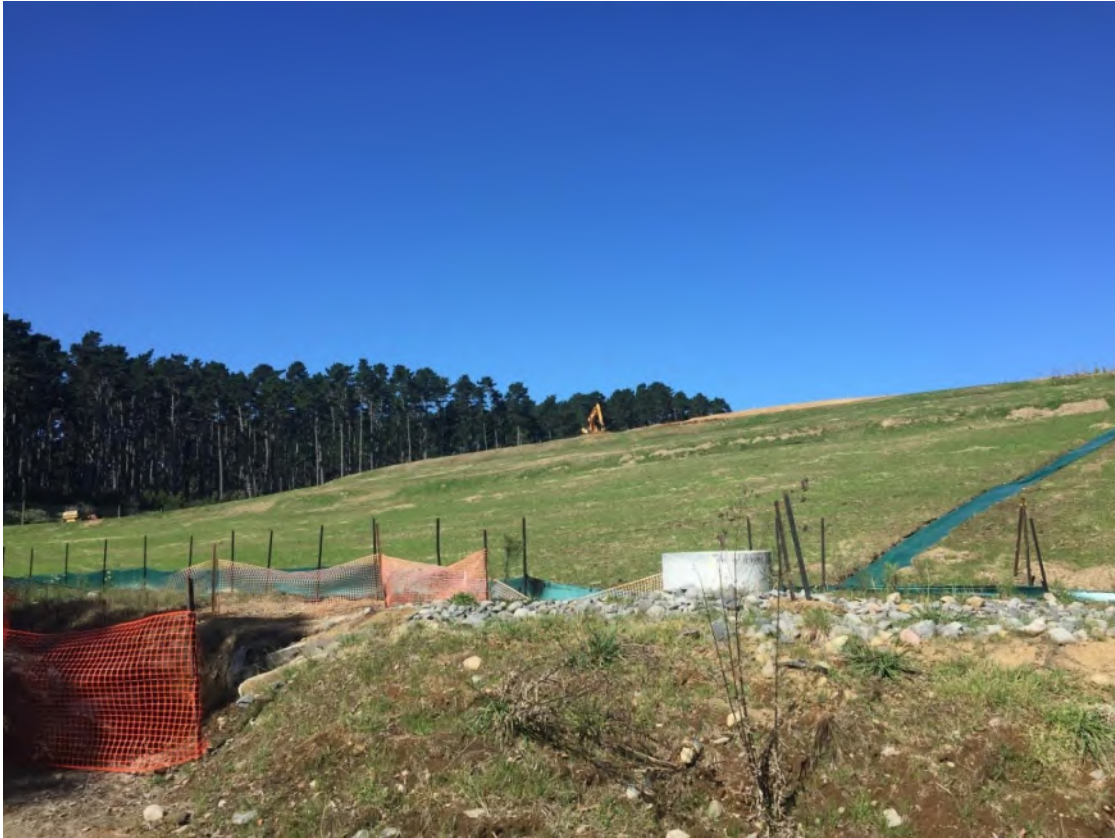
Photo 1 Finished and partially stabilised cap on the northern batter of Stage 3, April 2021
