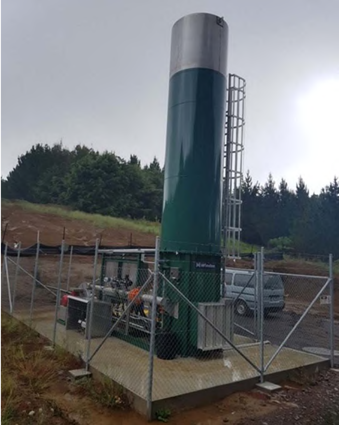
Photo 9 The fully enclosed flare
