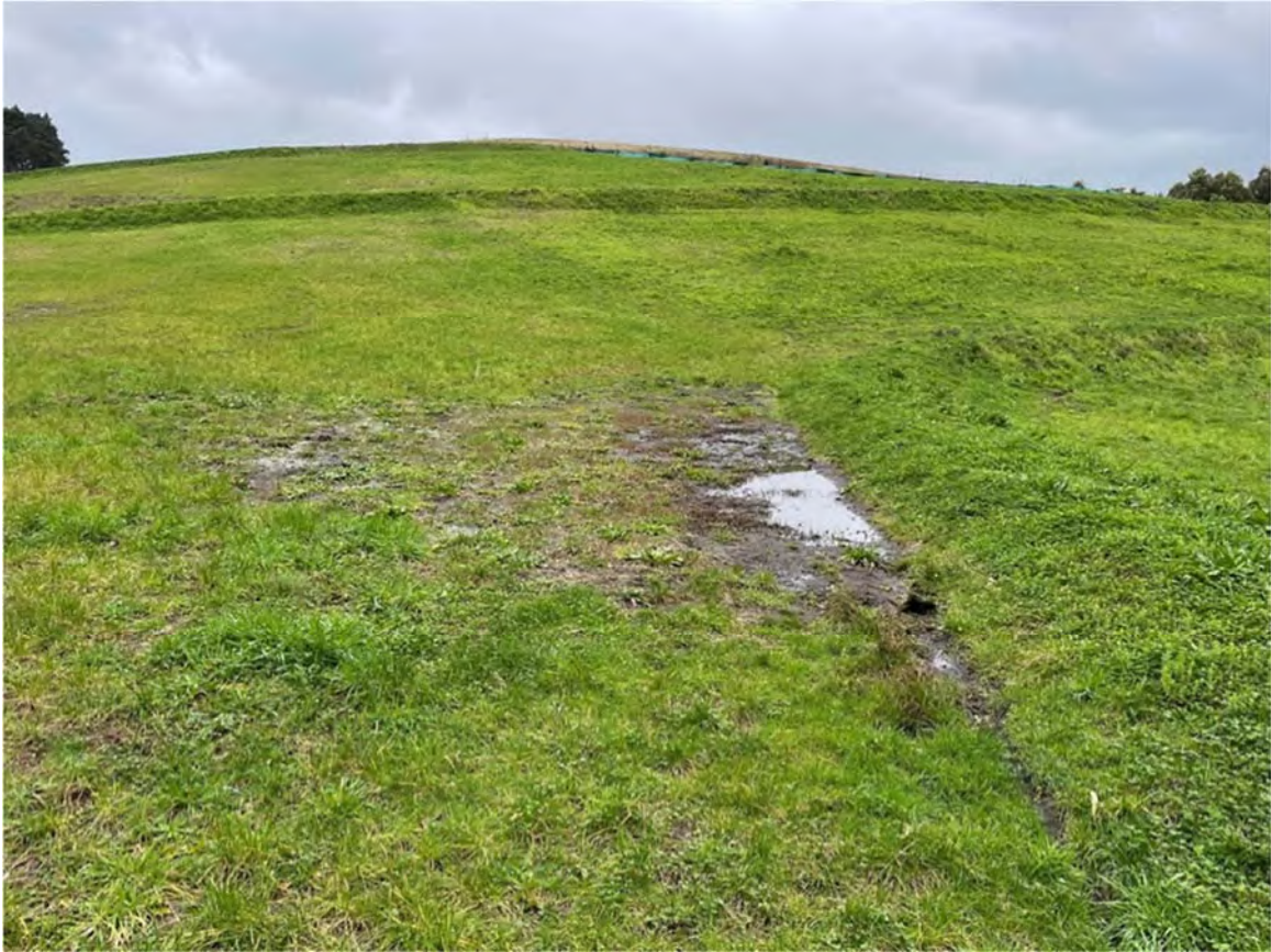
Photo 14 Small area of ponding, 19 July 2022
