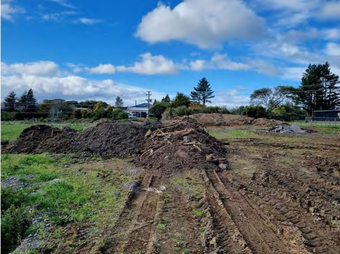
Photo 4 Fresh cleanfill material had been discharged to the unconsented site on the neighbouring property, 28 May 2024
