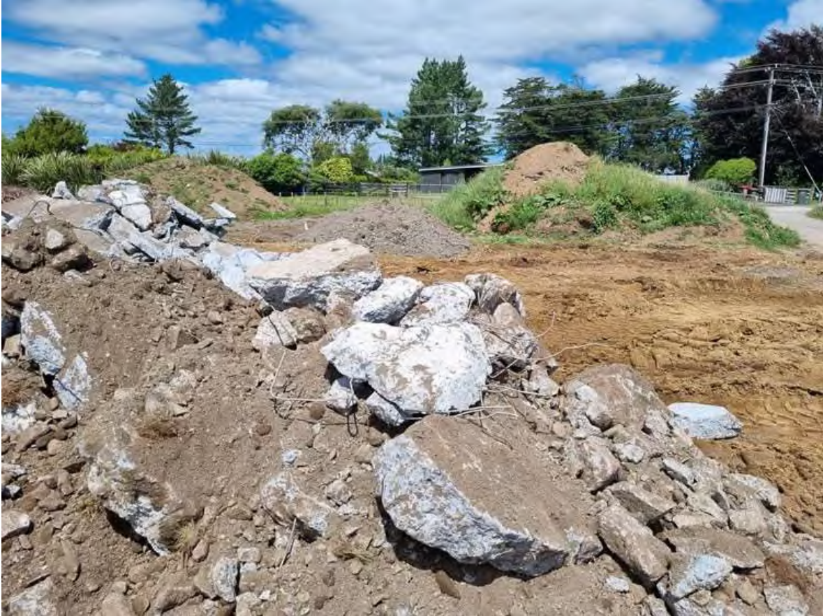
Photo 3 Cleanfill material discharged to an unconsented area of the neighbouring property, 14 February 2024
