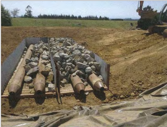
Photo 2 Example of a partially-constructed VUMU flarepit, such as was installed at Te Kiri North-A (courtesy of Todd Energy Ltd, 2014).
