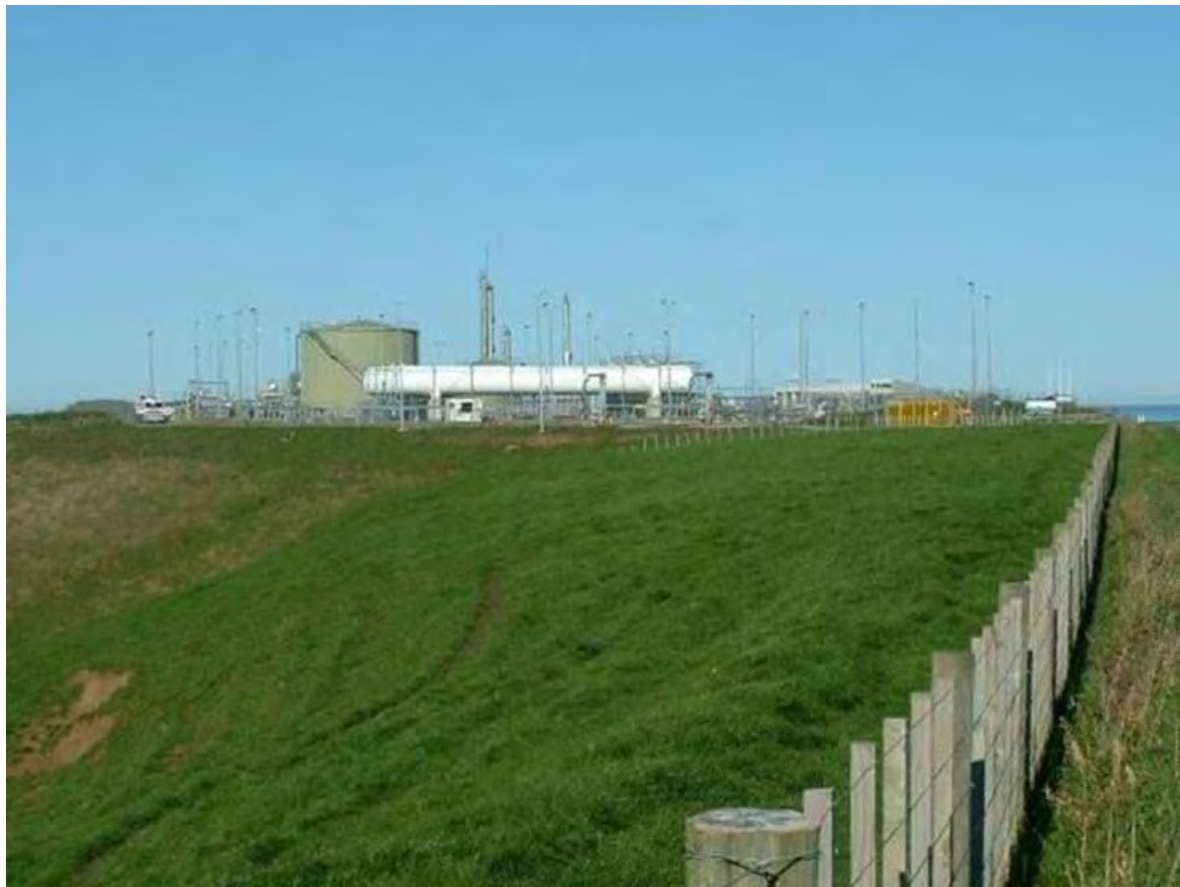
Photo 1 Rimu Production Station
