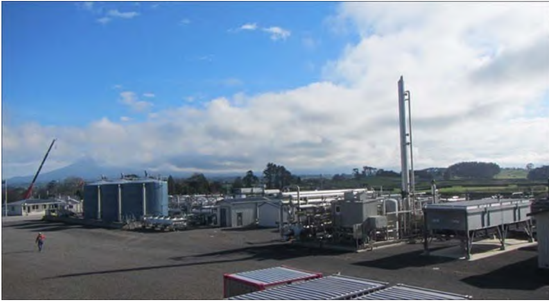
Photo 1 Cheal Production Station
