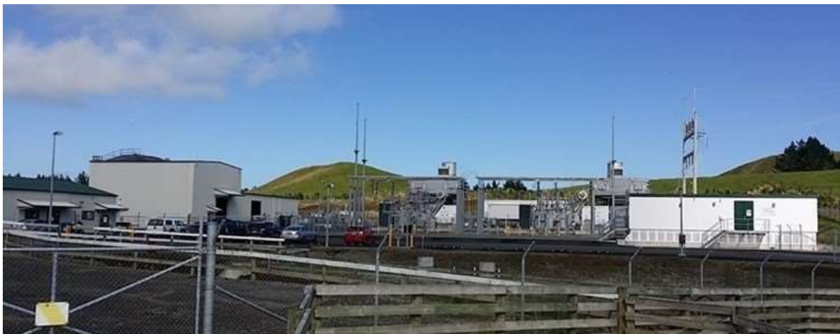
Photo 1 McKee Power Plant
