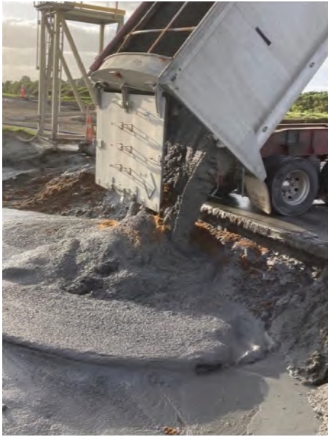
Photograph 1 – Discharge of cuttings and sawdust into Pit 1
