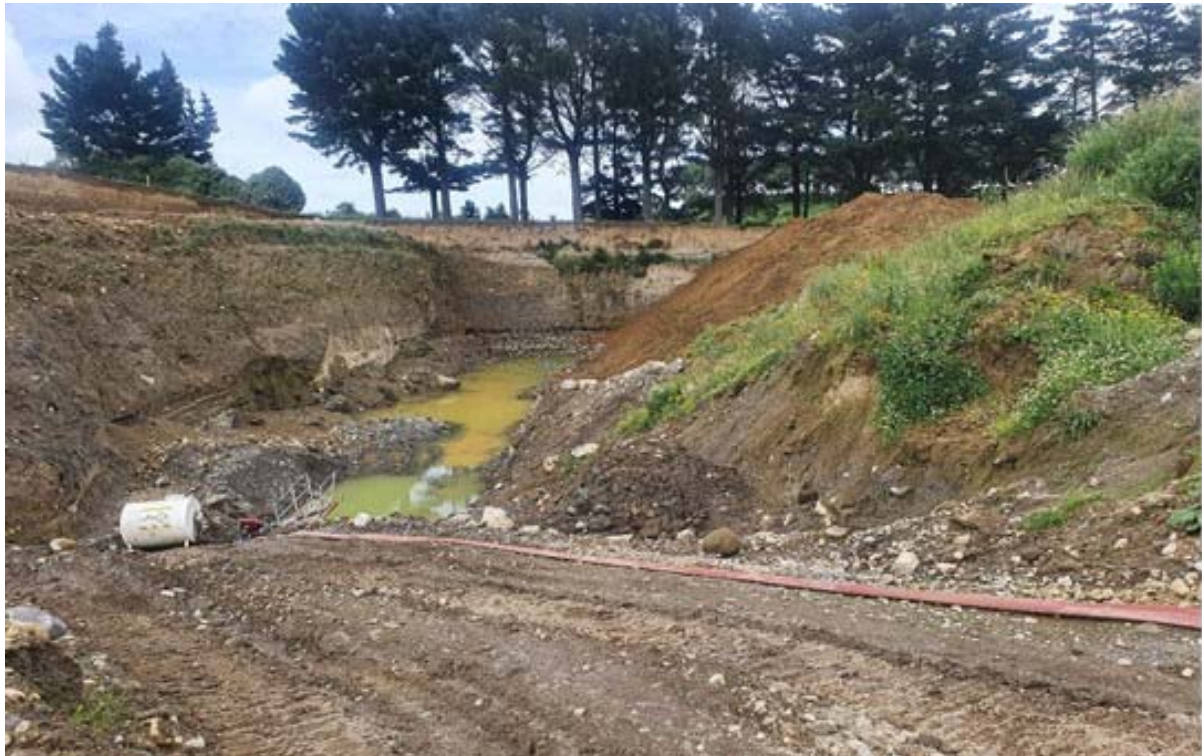
Photo 5 Active excavation site with groundwater present, pump to settling ponds also present.
