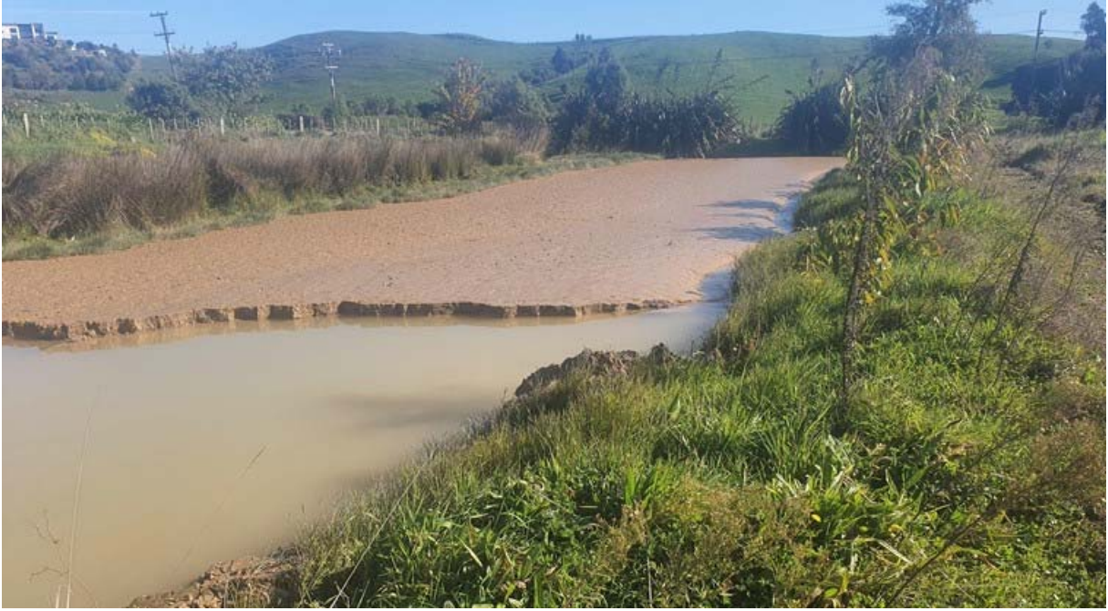
Photo 10 Ferndene Quarries Ltd, settlement pond requiring cleaning out, May 2022.
