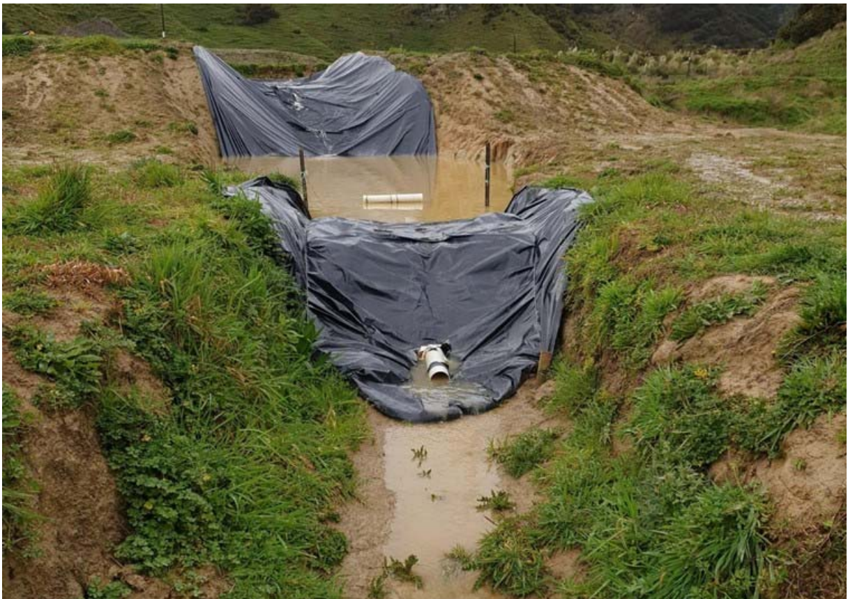
Photo 22 Uruti quarry settlement ponds for runoff from the new laydown area beside Mokau Road, October 2019
