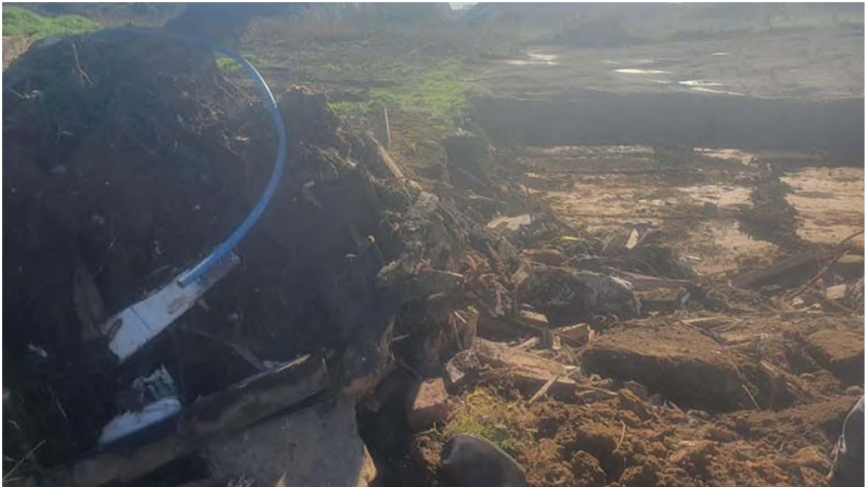
Photo 13 Ferndene Quarries Ltd, unauthorised cleanfill material, 12 th May 2022
