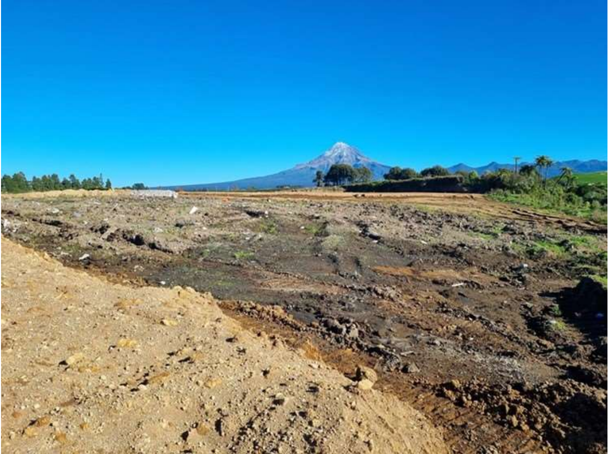
Photo 6 Ferndene southern cleanfill discharge area was in the process of being contoured, 8 May 2024
