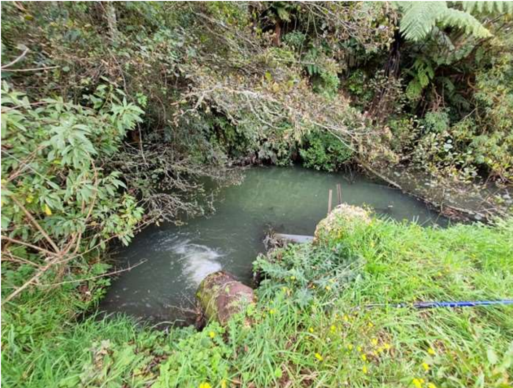
Photo 6 Final Pond F before the water flows through a culvert and into the unnamed tributary of the Kurapete Stream, April 2024
