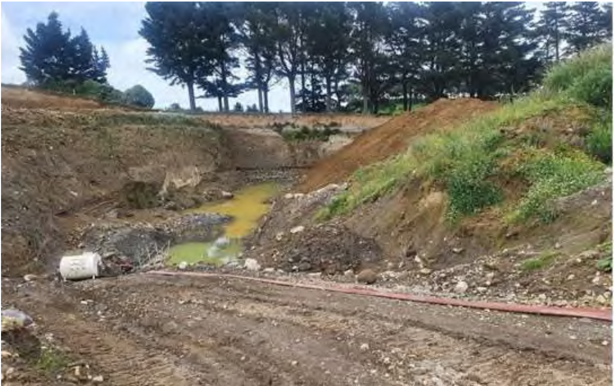
Photo 4 Active excavation site with groundwater present, pump to settling ponds also present
