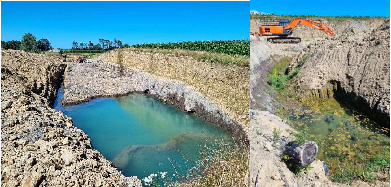
Photo 6 Hey Trust Quarry settling pond (left) looking toward open ring drain system as of January 2024. Settling pond (right) discharging to Kahouri Stream and/or the unnamed tributary
