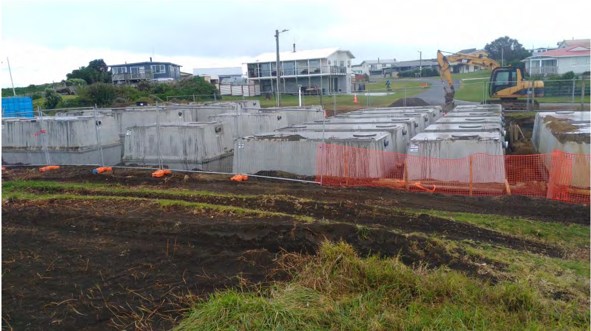
Photo 1 Construction of the SAF plant at the Waiinu Beach Settlement wastewater treatment system (Photo supplied by STDC)
