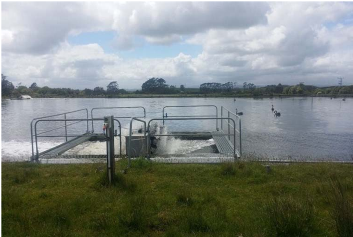
Photo 3 View of Stratford WWTP primary pond with aerators operating
