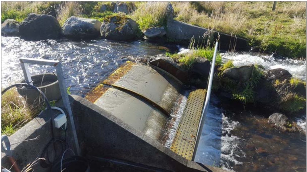
Photo 1 CCCWSL's weir and intake screen
