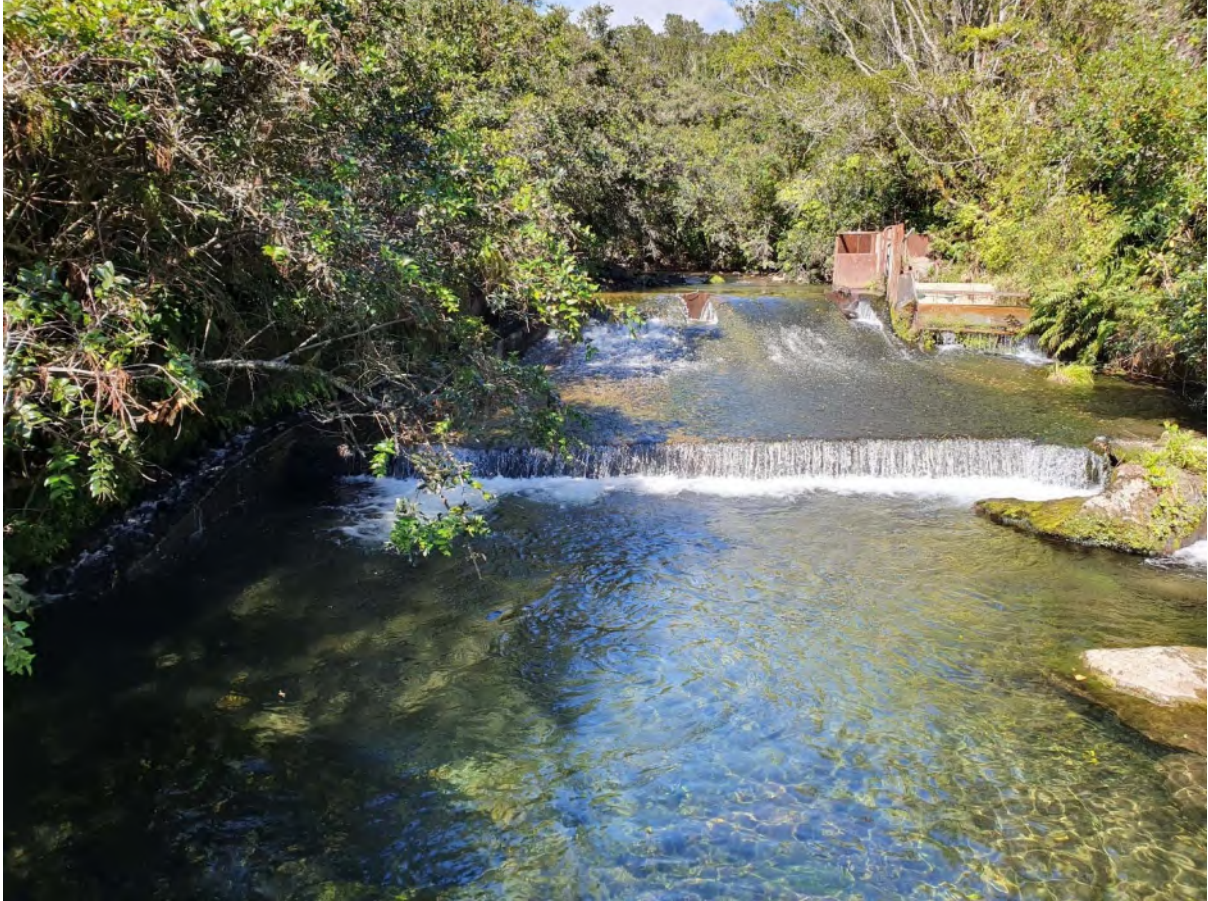
Photo 2 Ngatoro Stream weir and fish pass
