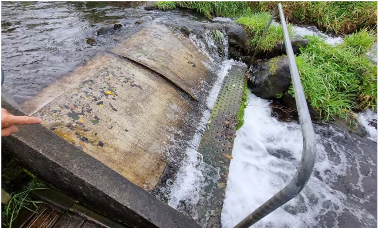
Photo 1 CCCWSL's weir and intake screen
