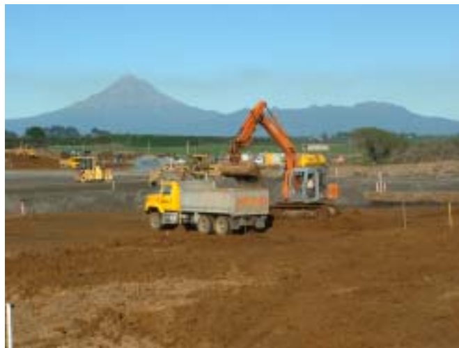
Photo 1: Water from cleaning earthmoving equipment must not enter the stormwater drains
