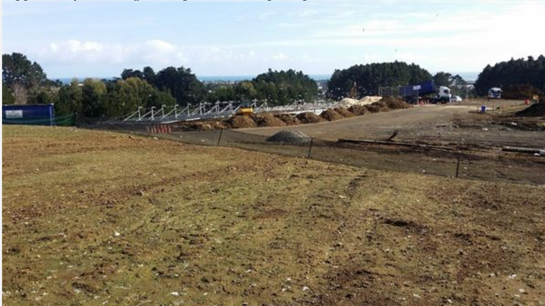
Use of metal covers to provide adequate daily cover that operators can manage efficiently, supported by confining the disposal to a compact operational area.
