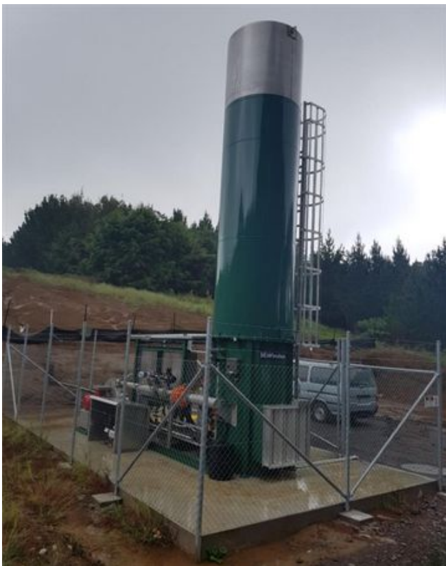
Photo 3 The fully enclosed flare
