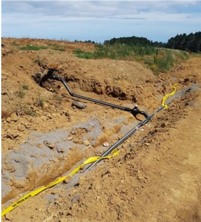
Photo 2 Leachate pipes feeding into the gas collection system
