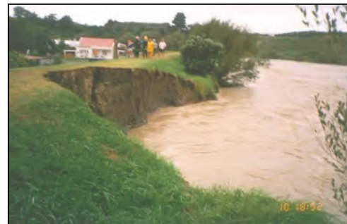
Figure 3: Waitara River bank collapse – 1990
