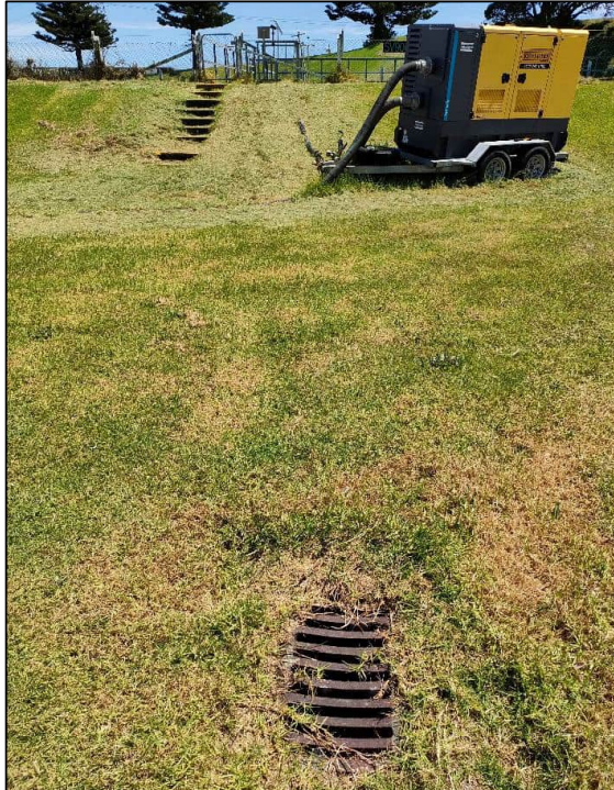
Photograph 6: Pumps servicing the stormwater ponds SV9000/9100.
