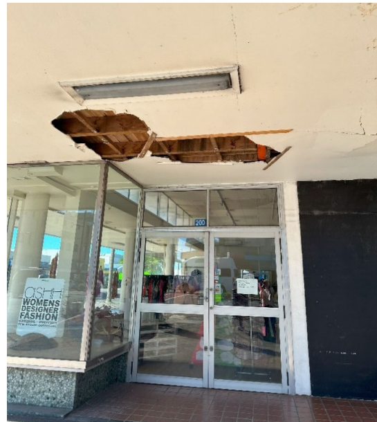
Main Street building decay. Gladstone Rd
