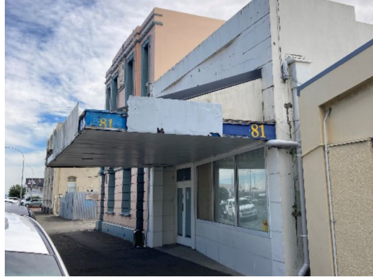
Deteriorating building. Childers Rd
