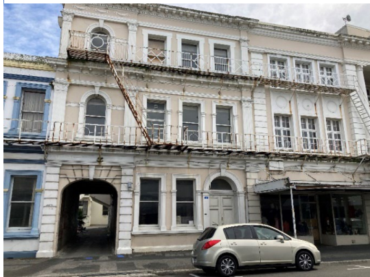
Masonic Hotel decaying façade. Lowe St
